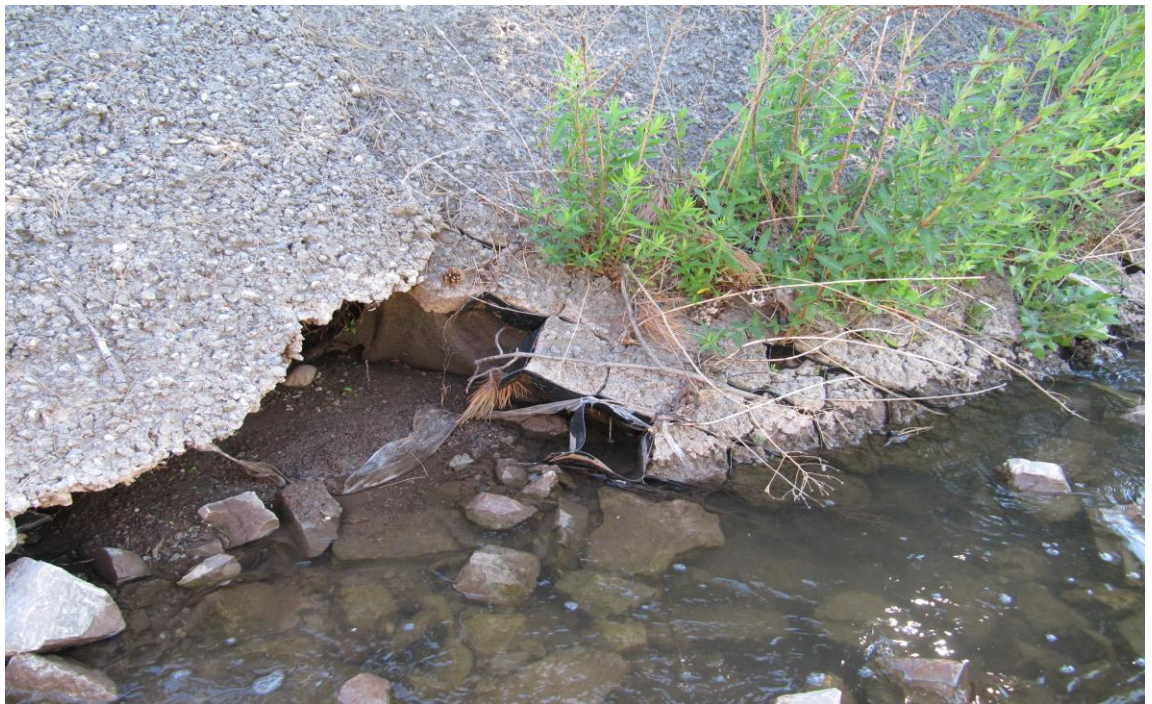
Scour of Streambed – Note Exposed Geogrid near Outlet
