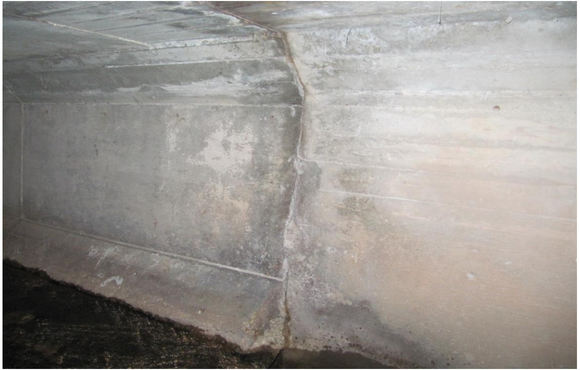
Concrete Disintegration at the Drop-off Location
