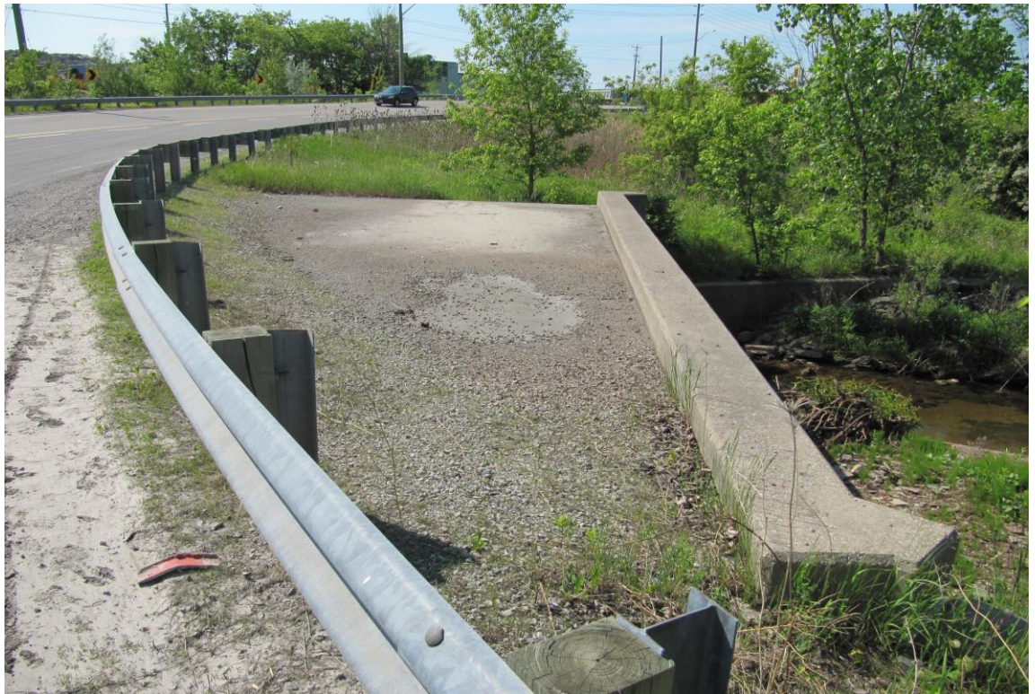
Condition of Existing Guide Rail System
