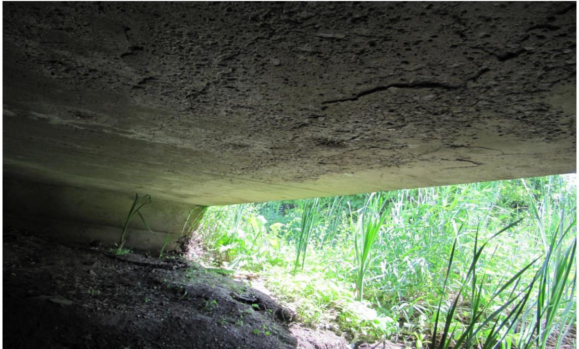
Concrete Honeycombing near Outlet
