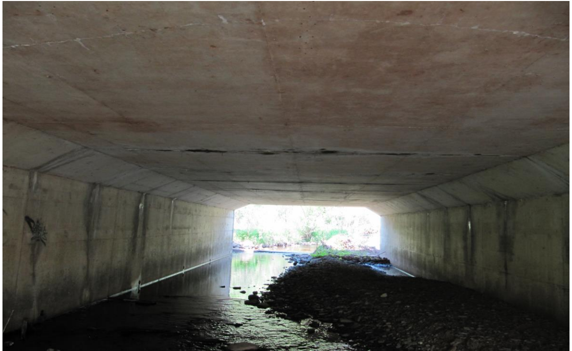
Sediment Buildup in the South Cell Looking West
