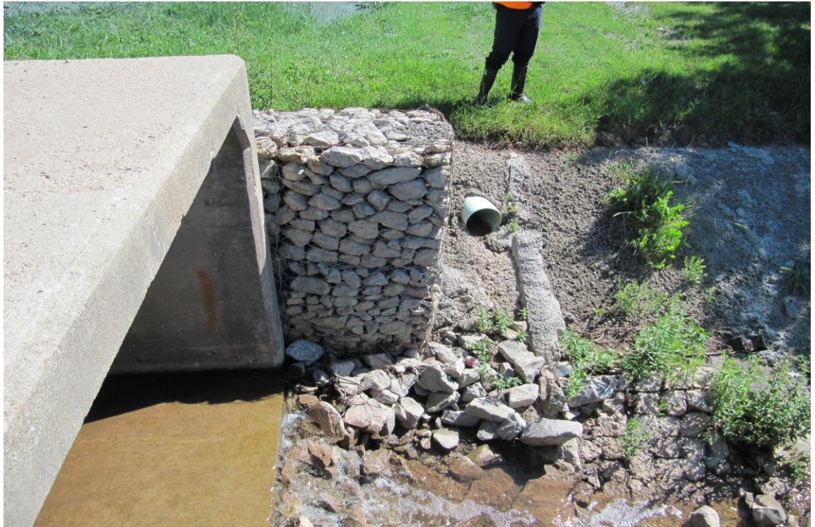
Condition of Gabion Basket
