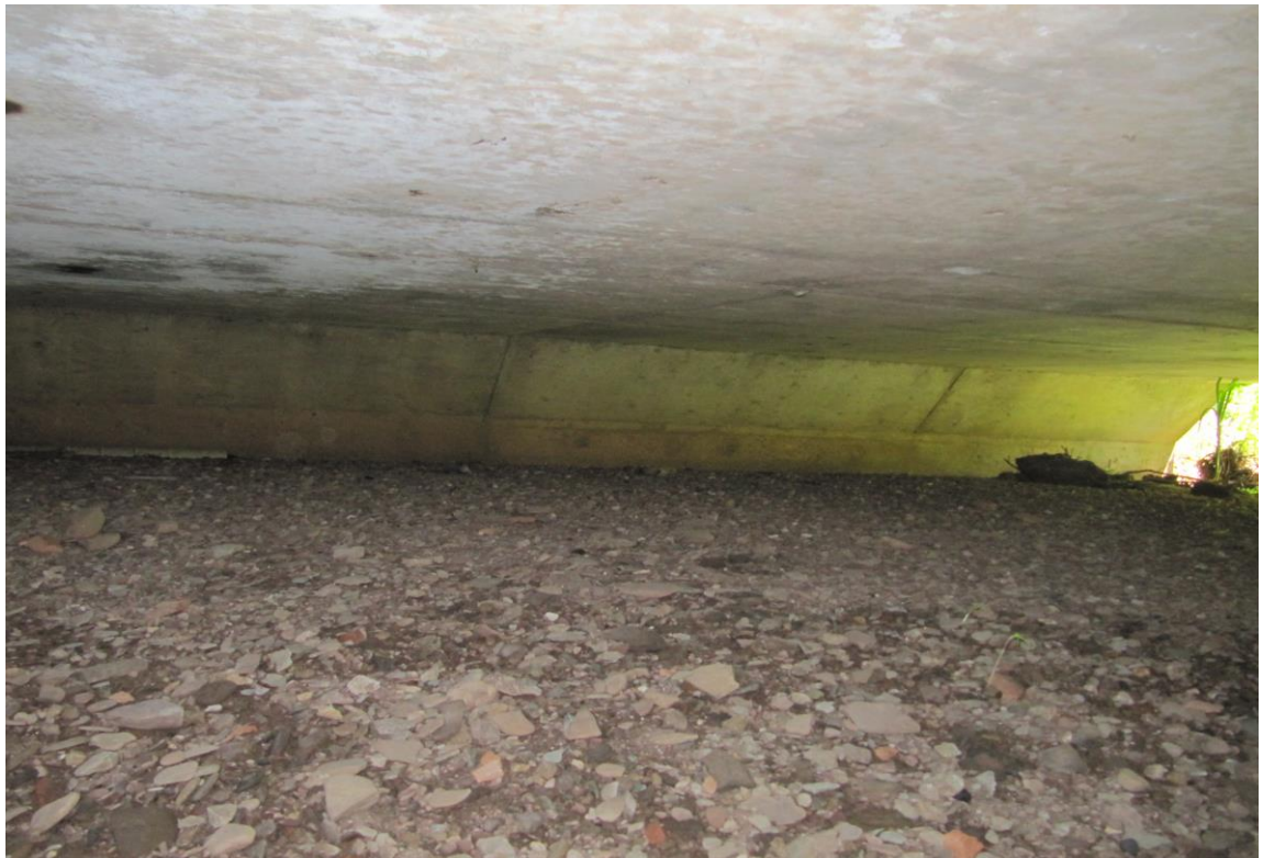
Heavy Sediment Buildup inside the Structure
