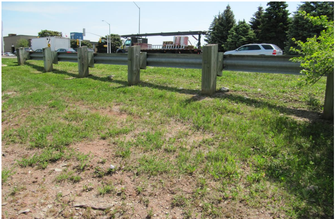
Condition of Existing Guide Rail System
