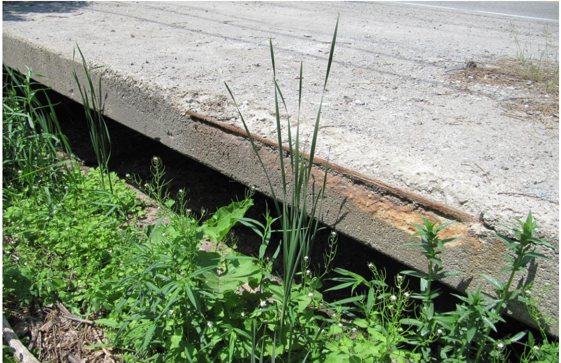
Spalled Concrete with Exposed Rebar at Outlet
