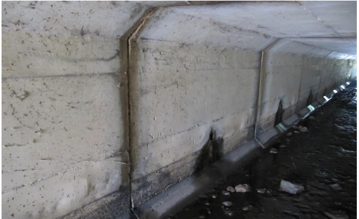
Transverse Separation of the Concrete Segments
