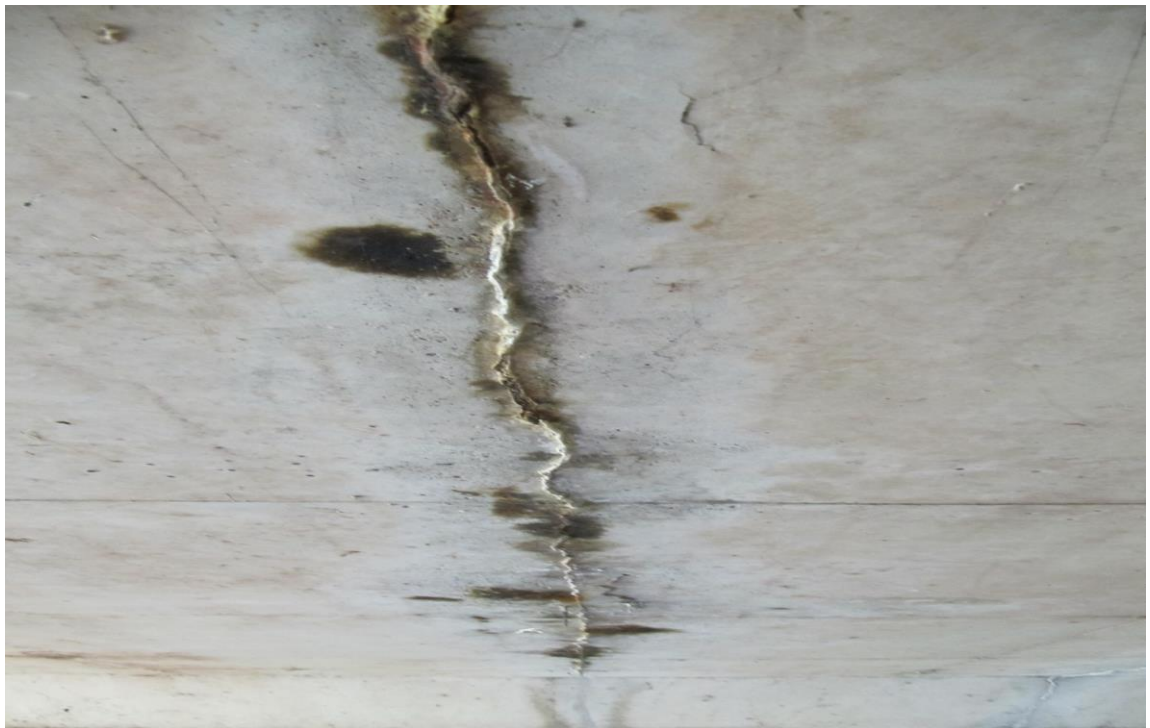
Transverse Crack in the South Cell (Typical)
