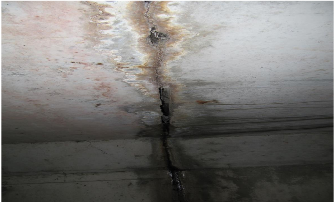
Concrete Spalling and Delamination
