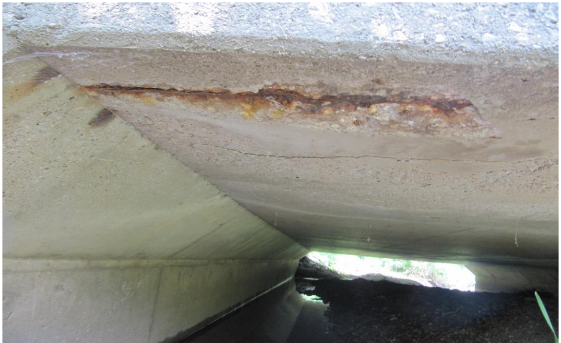
Spalled Concrete with Exposed Rebar of Soffit near Outlet
