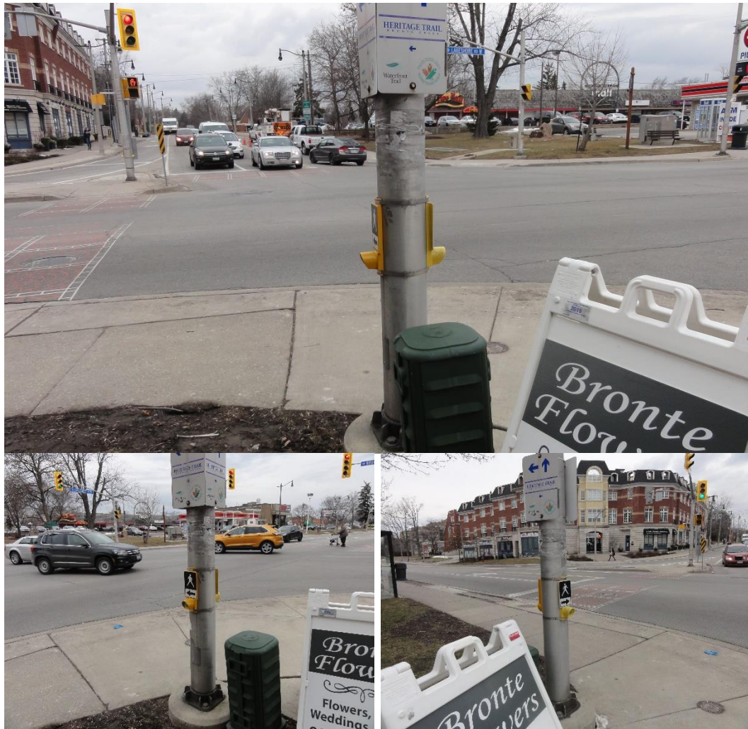
FIGURE 14: Confusing Placement of Pedestrian Pushbuttons
