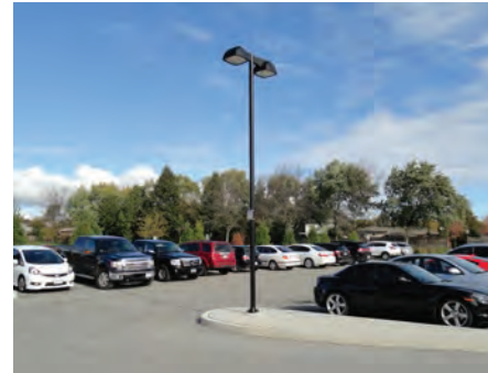
Full cut-off fixtures direct light downward to prevent spillage (4.4.5)
