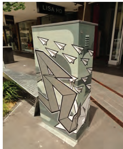
Above ground utility box creatively concealed (2.2.22)
