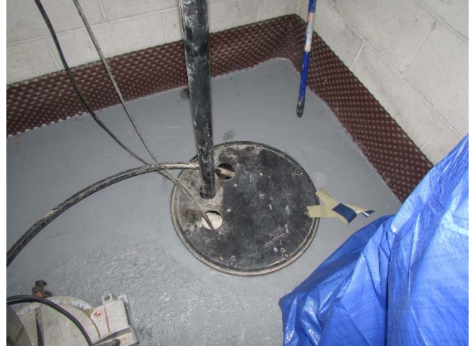
Photo 10: View of a sump pit in the basement of Building C at the time of the site reconnaissance.
