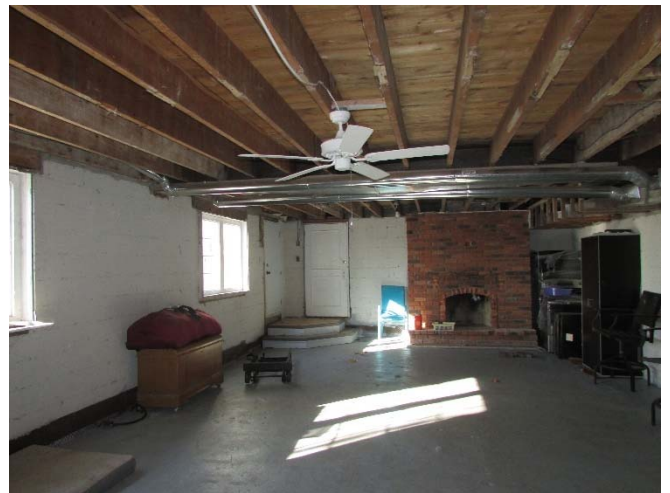
Photo 12: View of a portion of the basement of Building A at the time of the site reconnaissance.
