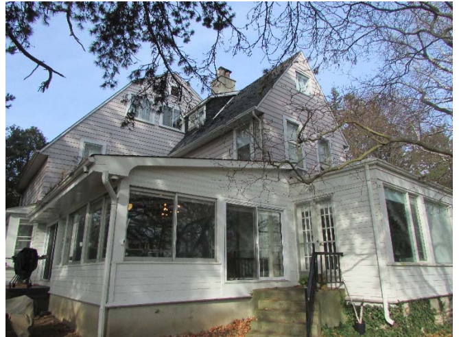
Photo 4: View of a portion of the south elevation of Building C, looking north.
