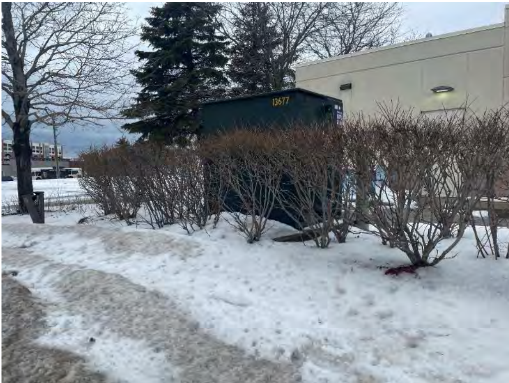
Photo 18: Transformer located at 562 Trafalgar Road, approximately 170 m east.
