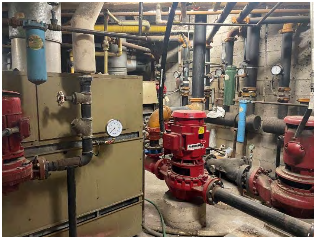
Photo 8: Mechanical room in Site building.
