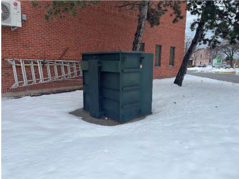
Photo 3: Transformer located on-Site to the west of the Site building, facing southeast.
