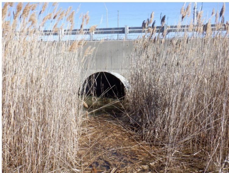
Photo 6-2 Looking east from the west side of Bronte Road, south of Highway 407, at the existing culvert that conveys Stream Reach 14E-8
