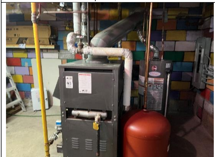
5. View of the boiler room in the sub-basement of 304 Spruce Street.
