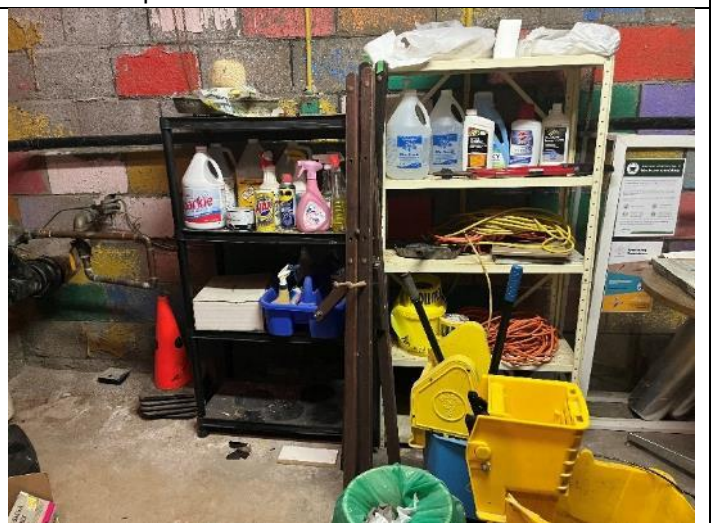
6. Small quantities of household cleaners observed in the boiler room of 304 Spruce Street.
