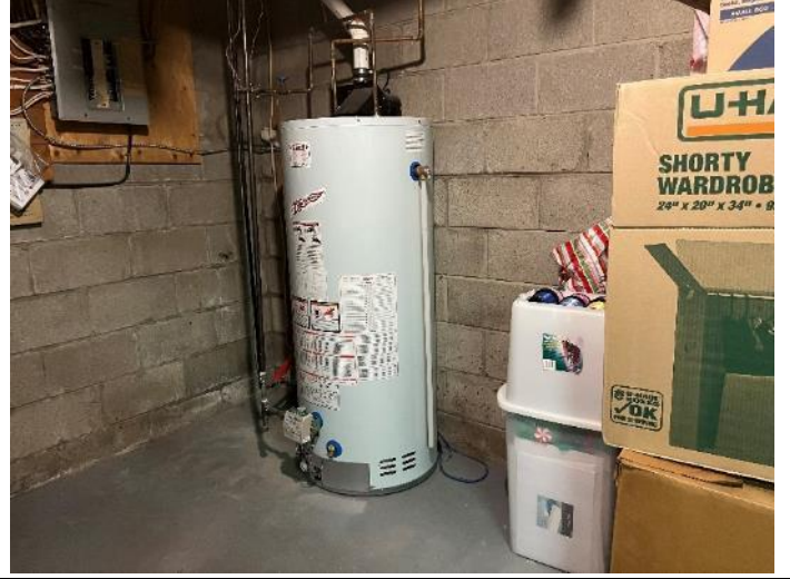
10. Hot water tank in the boiler room of 318 Spruce Street.
