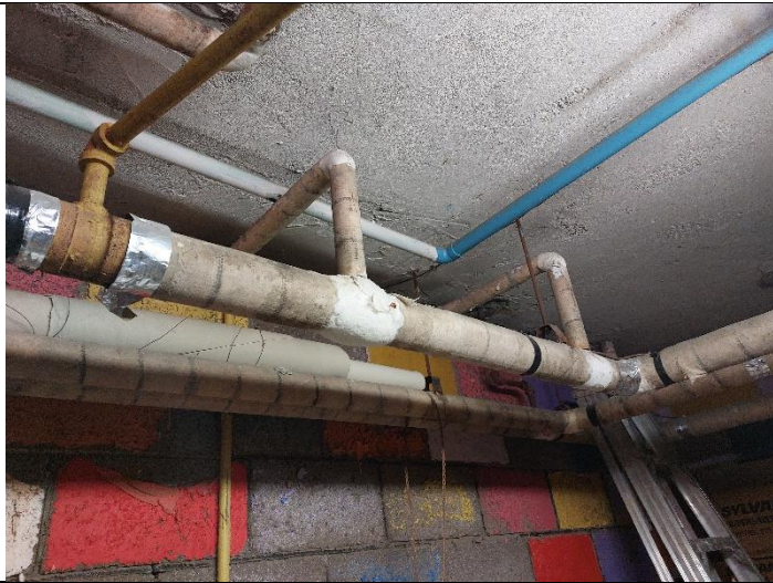
7. Potential presence of asbestos as pipe insulation in the boiler room of 304 Spruce Street.
