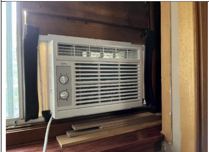
3. View of the wall-mounted cooling unit observed in the office area of 304 Spruce Street.
