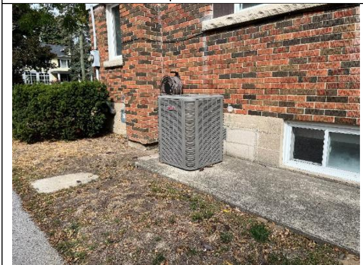
17. Air-conditioning unit, located on the west exterior wall of 318 Spruce Street.
