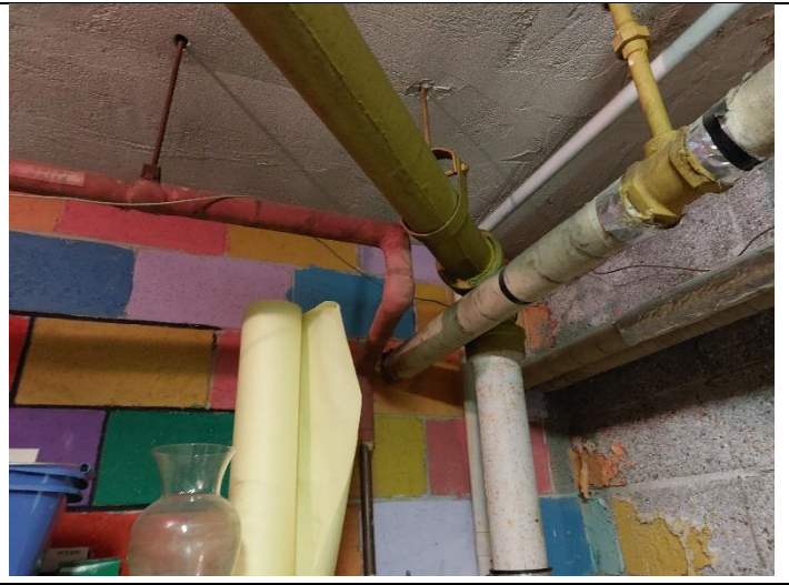
8. Potential presence of asbestos as pipe insulation in the boiler room of 304 Spruce Street.
