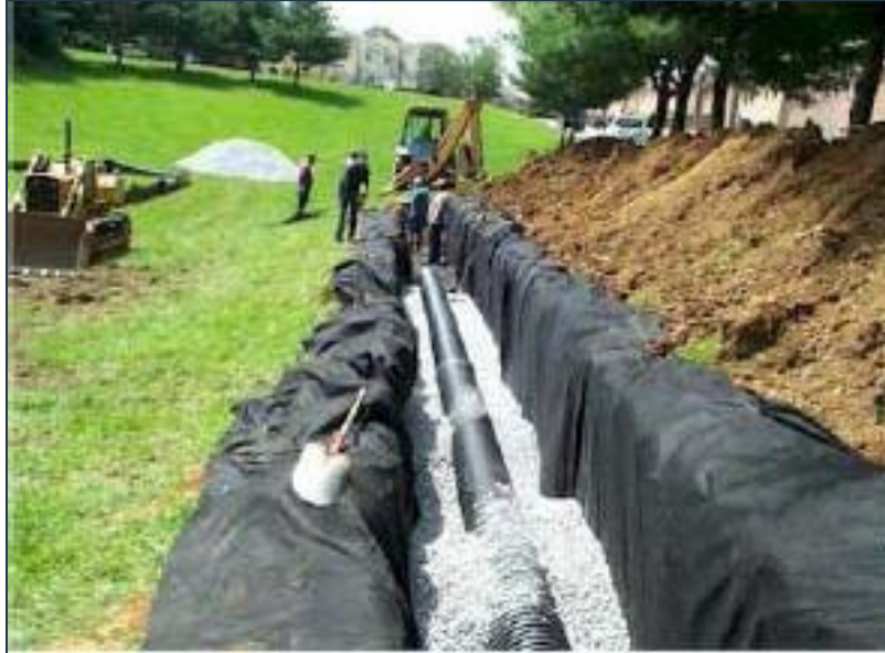
Figure 7-14: Infiltration Trench Construction (Low Impact Development Stormwater Management Planning and Design Guide, Version 1.0, CVC and TRCA, 2010)
