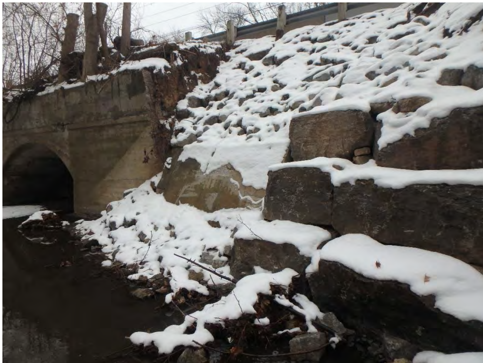
Photo 12: Emergency works were completed in the summer of 2017 to repair the severely eroded bank present directly west of the Lakeshore Road crossing.
