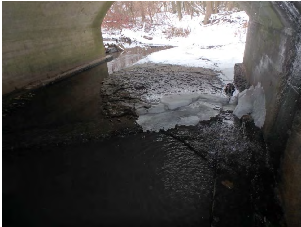
Photo 14: Standing within Lakeshore Road ROW facing upstream. Note large area of limestone present to right (east) of structure inlet. Cement slab located at left may pose a potential barrier to smaller-bodied fish during periods of high flow.
