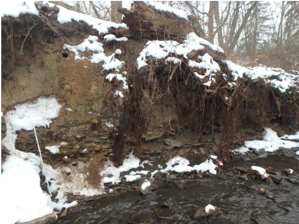
Photo 11: Bank nearest the retaining wall structure experiencing significant erosion. Erosion of bank reaches approximately 2.5 meters in height at its highest point.
