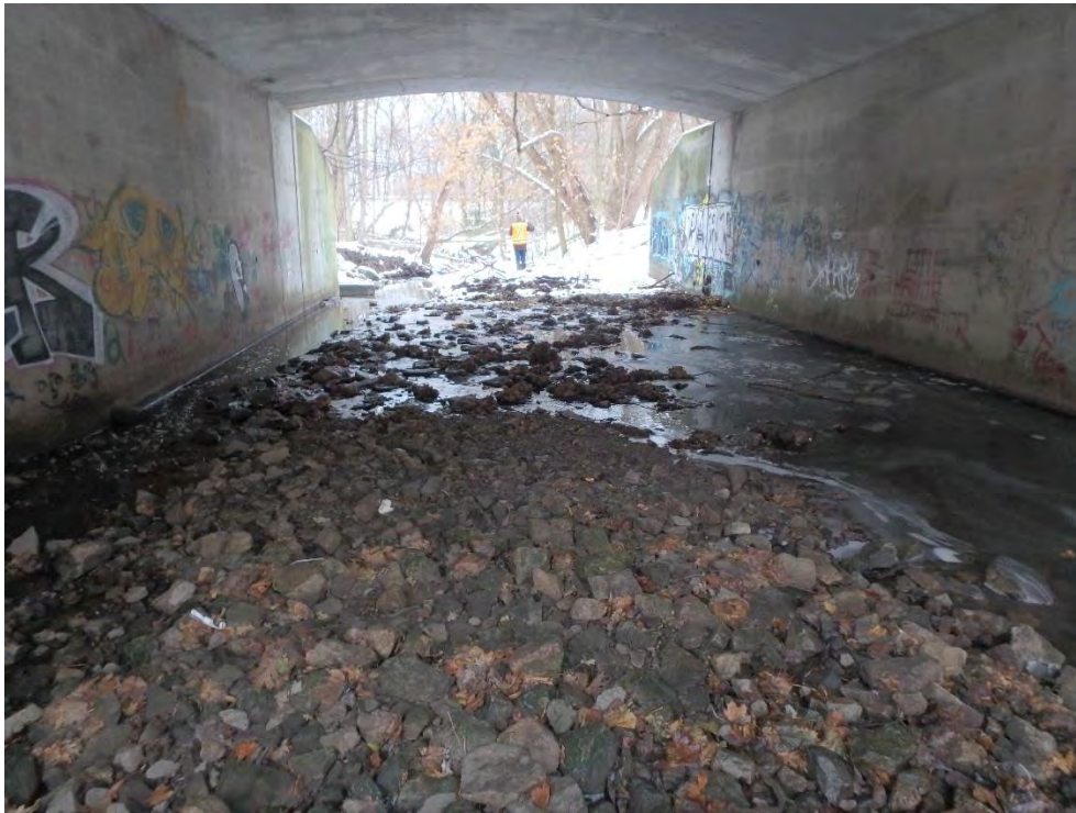
Photo 1: Within Rebecca Street ROW facing downstream. Note large area of debris at west downstream end of crossing forcing flows to move over cement ledge on east.
