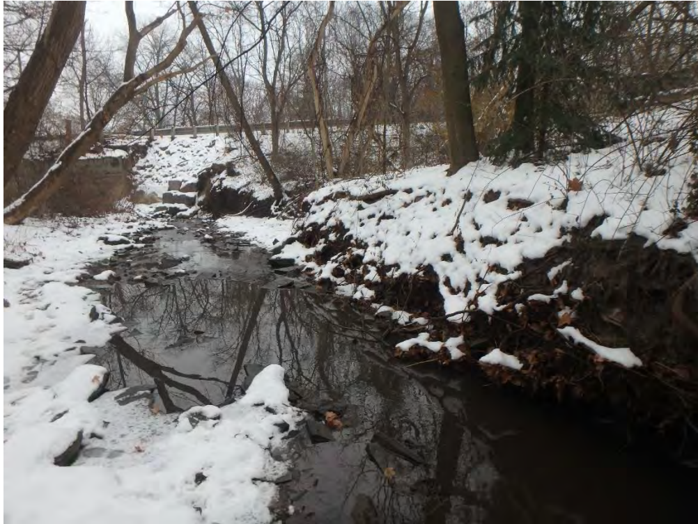
Photo 9: Erosion evident at west bank on approach to Lakeshore Road ROW.
