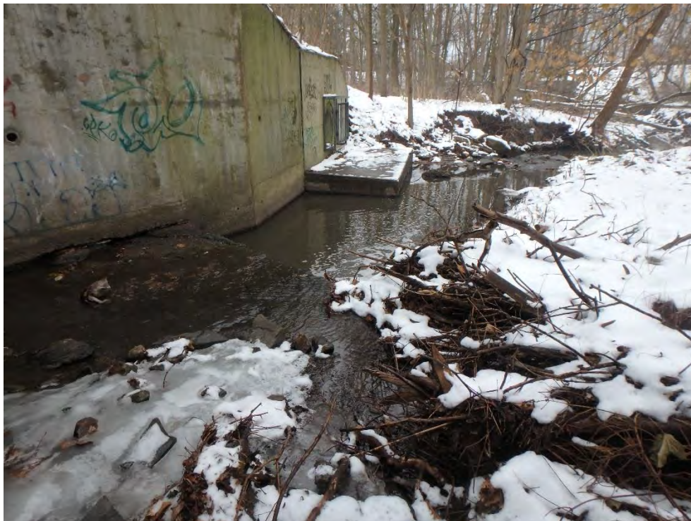
Photo 2: Cement slab present at downstream end of Rebecca Street crossing is a barrier to small-bodied fish.
