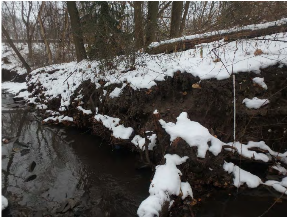
Photo 8: Erosion evident on west bank for approximately 31.5 meters prior to reaching retaining wall for Lakeshore Road.
