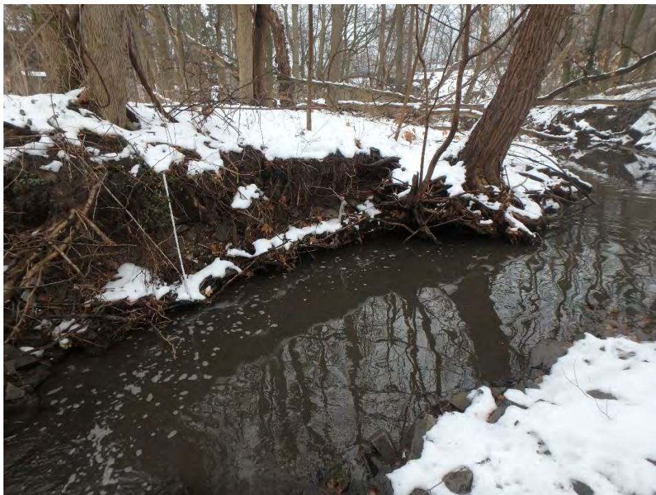
Photo 6: Erosion evident at east bank immediately downstream of Rebecca Street retaining wall.
