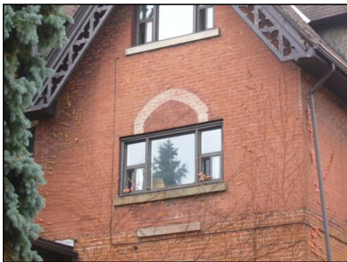
Window sizes and shapes should be retained and the example above avoided.
