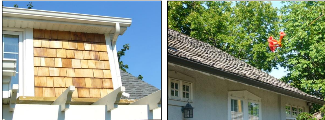
The appropriate use of traditional materials such as brick, wood siding and wood shingles, as shown above, is encouraged.
