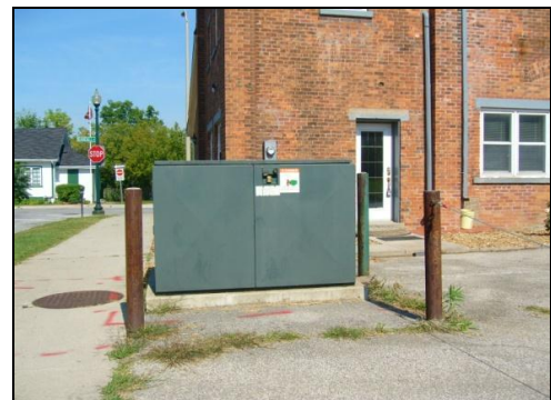
Utility boxes and coverings, such as this transformer box, should be screened.
