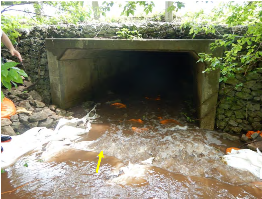
Immediately upstream of the ~100 m long culvert conveying flows across the QEW and the South Service Road, sand bags spanned the channel creating a weir.
