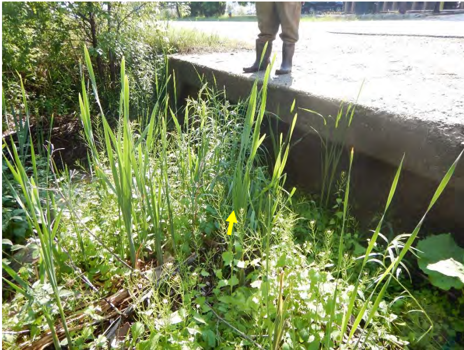
A well-vegetated bar blocked approximately two-thirds of the Wyecroft Road culvert outlet, on the eastern side.
