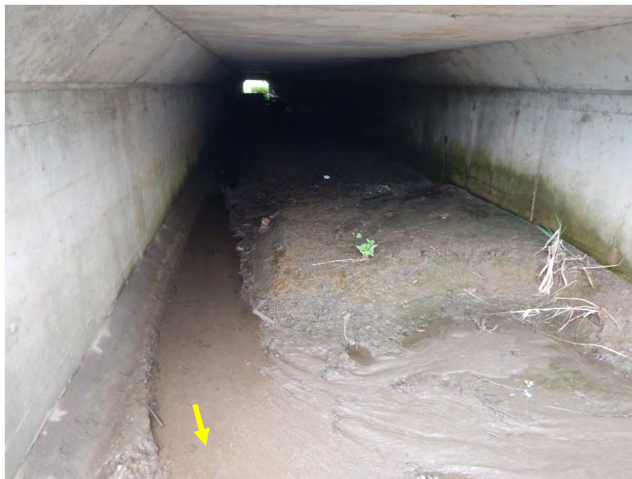
Sediment has accumulated within the eastern culvert, with a narrow and shallow channel along the west side of the culvert.
