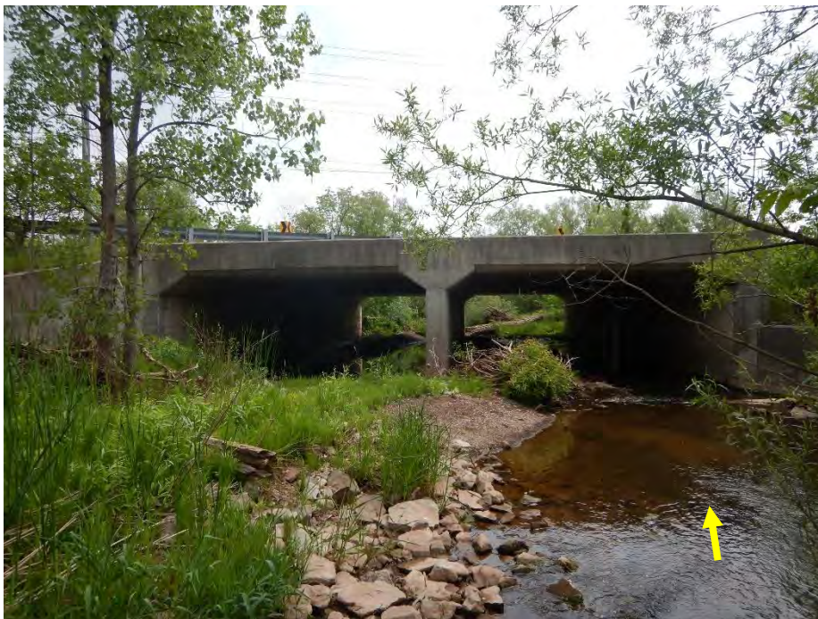
The South Service Road crossing was a twin box culvert, with the channel aligned with the southern culvert. The northern culvert was partially blocked by a well-vegetated bar.
