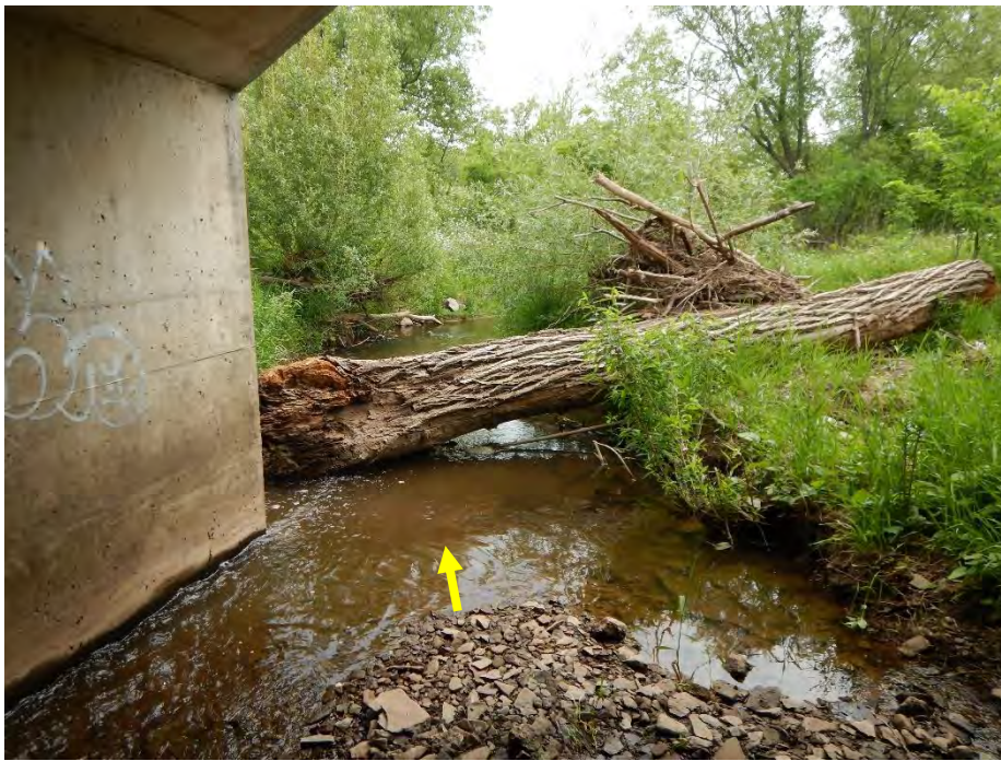
The channel was naturally constricted at the downstream end of the southern box culvert. A fallen tree transverse to the channel further impeded flows.
