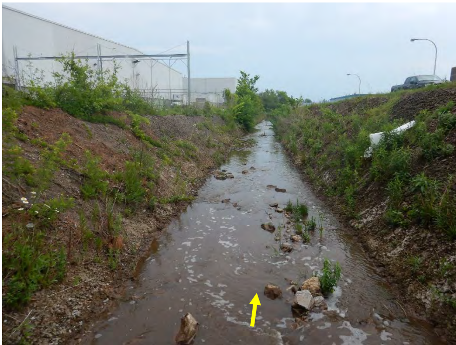
Downstream of South Service Road the channel was straight and concrete-lined with no morphological variability.
