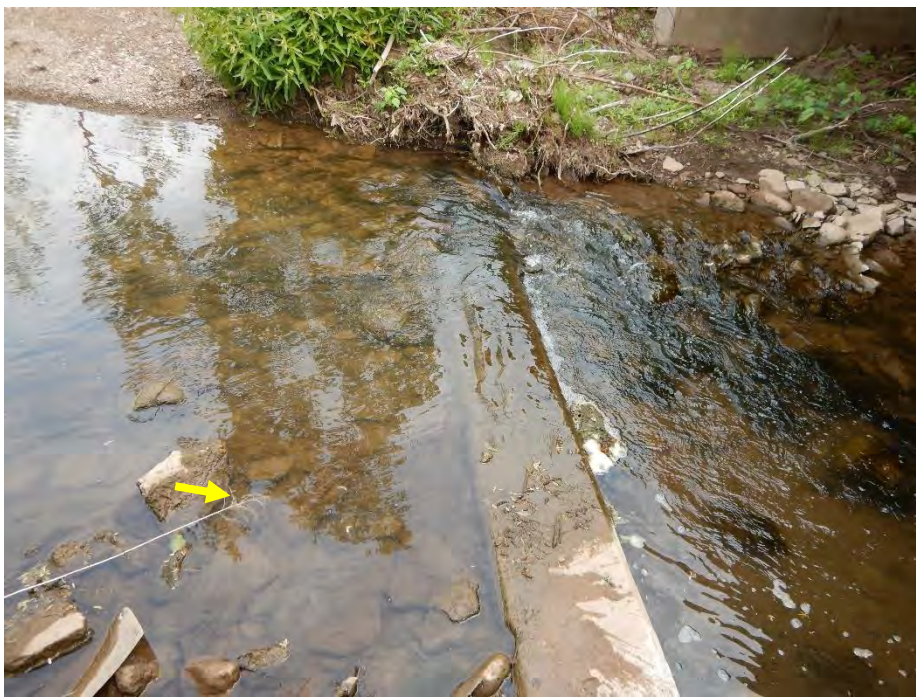
A concrete weir spanned the channel immediately upstream of the South Service Road crossing.
