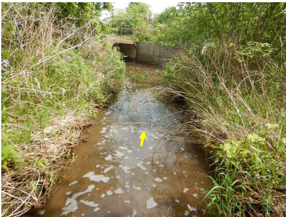
The channel bed and banks were lined with articulated concrete blocks throughout the extent assessed. No erosion was noted to channel bed or banks.
