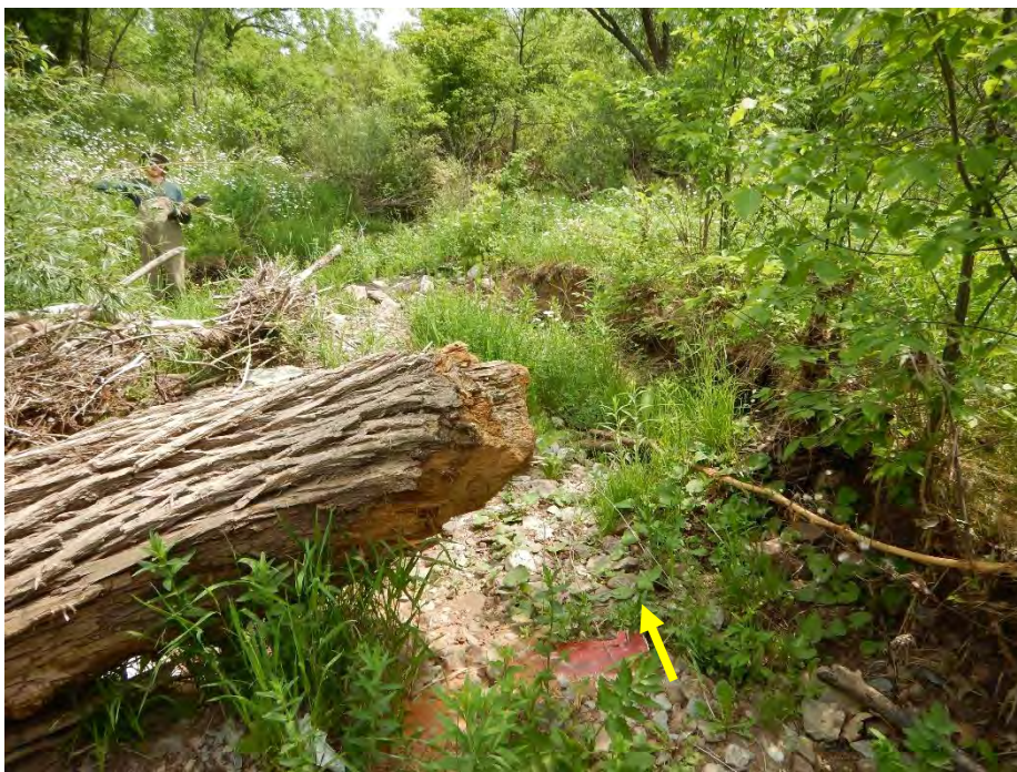
Due to the channel constriction beyond the downstream end of the southern culvert, high flows have evidently overtopped the bank and eroded the south valley wall.
