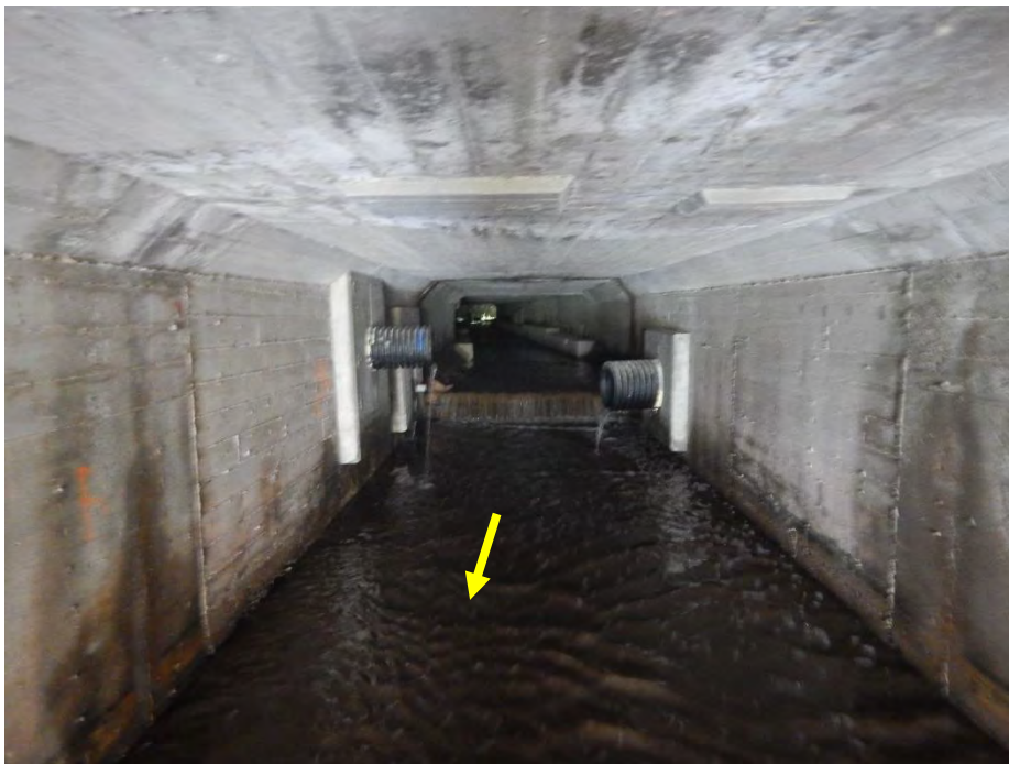
Within the culvert, two drops each approximately 0.3 m high were observed. These may prevent upstream fish migration.
