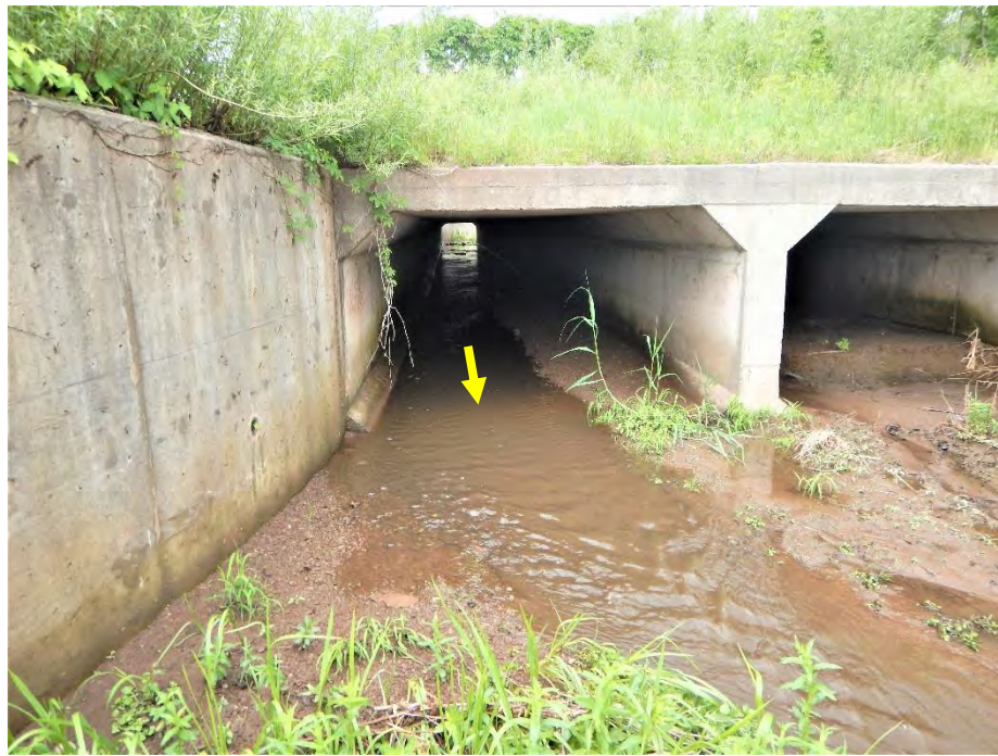
Within the western culvert, low-flow travelled along the west side of the culvert, and sediment was deposited along the east side.
