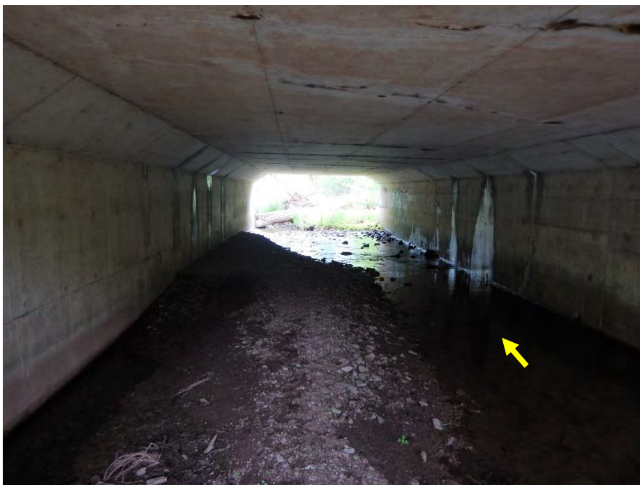
A bar formed along the north side of the southern box culvert.
