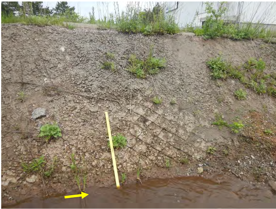
Channel banks were generally 2 m high and had a 1.5:1 slope, with some erosion from abrasion exposing the supporting wire within the concrete.
