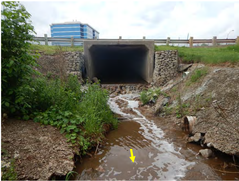
Another drop was present at the culvert outlet at South Service Road. The channel banks were composed of concrete, but eroded along the toe in the vicinity of the culvert outlet.
