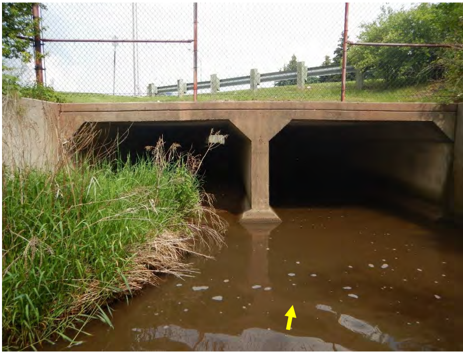
The South Service Road crossing was a twin box culvert. While both culverts conveyed flow, the eastern culvert was partially blocked by a well-vegetated bar. Two-metre-high concrete retaining walls directed flow into the culvert.
