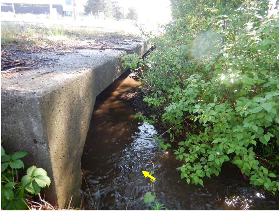
A well-vegetated bar blocked approximately three-quarters of the Wyecroft Road culvert inlet.
