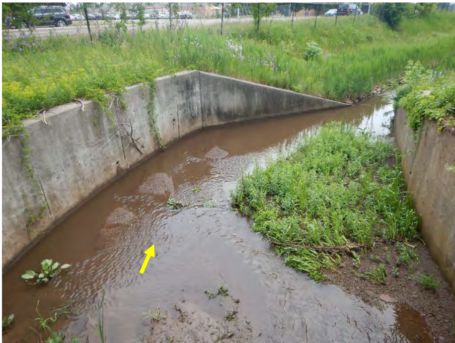
At the outlet of the South Service Road culvert was a vegetated bar.
