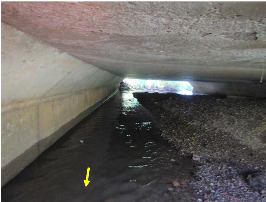
The channel makes a 90° turn upon entering the Wyecroft Road culvert before following the western wall to the outlet.
