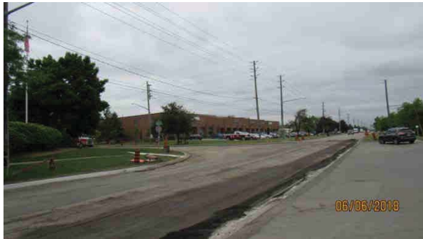
Plate 7: North view of Wycroft Rd at Westgate Rd.; Area is disturbed, no potential
