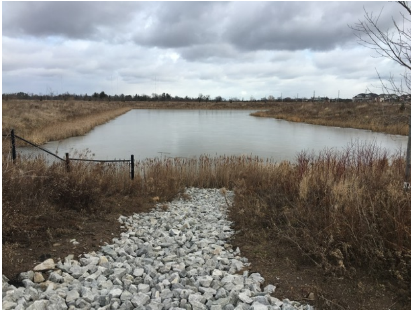
Stormwater management pond east of the Hospital, view facing east towards Sixteen Mile Creek
