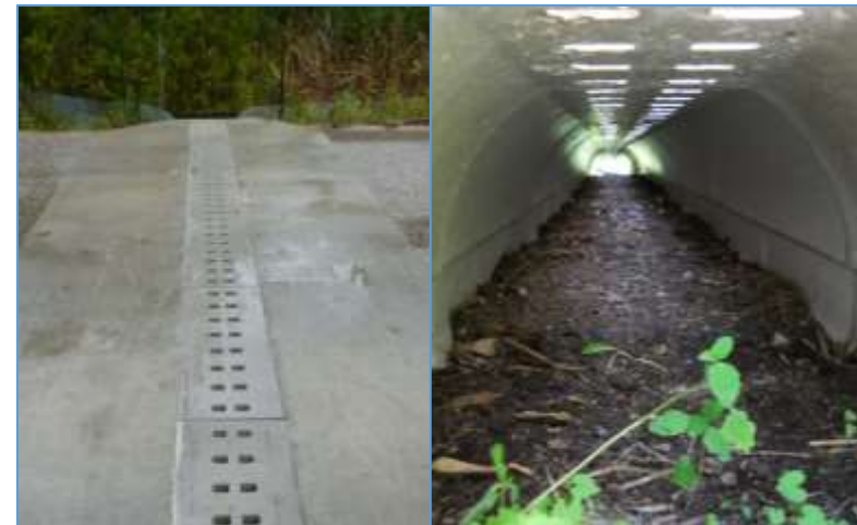
Ecopassages create safe a passage for animals crossing under roads
