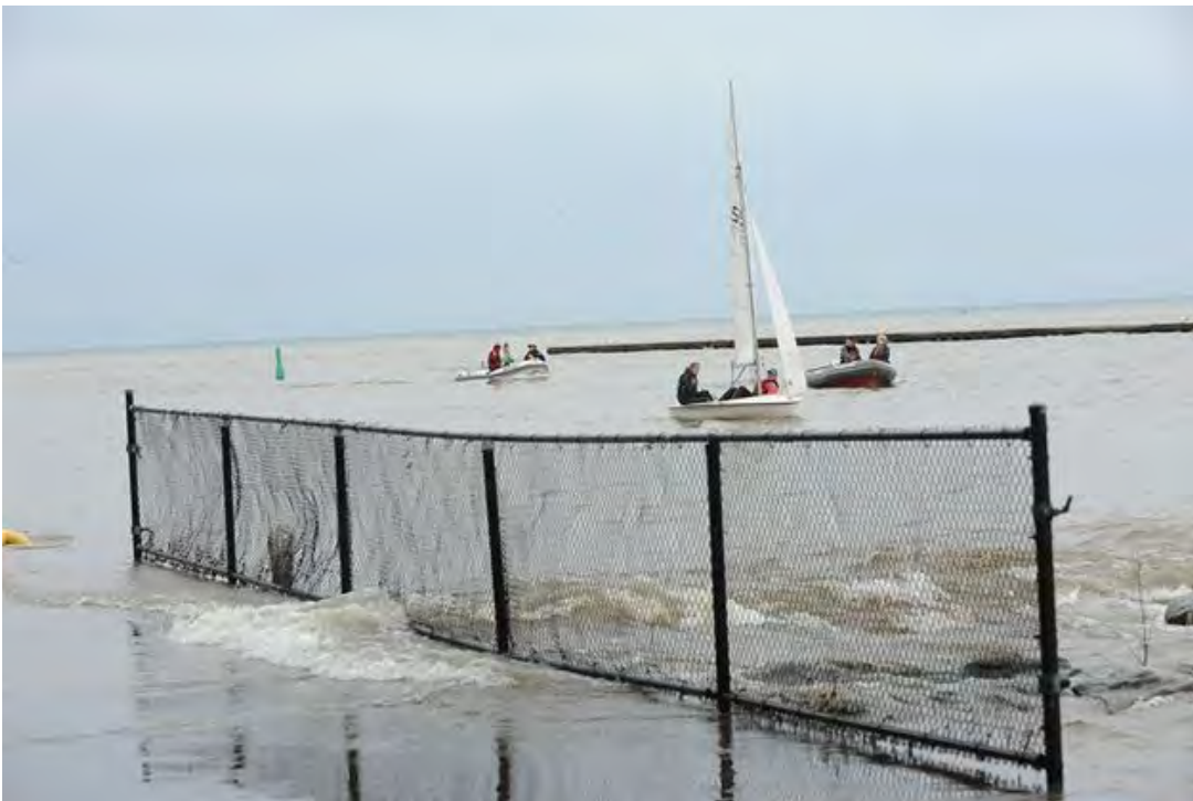
Figure 35: May 2017 photograph of water submerging the pier wall at Bronte Harbour (Source: Paine, 2017).
