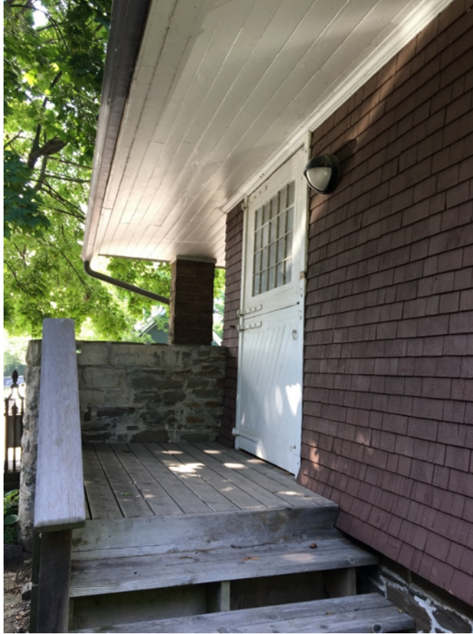
Figure 60: Coach House and Gardener's Cottage's manure pit wall and Dutchman door, west façade.
