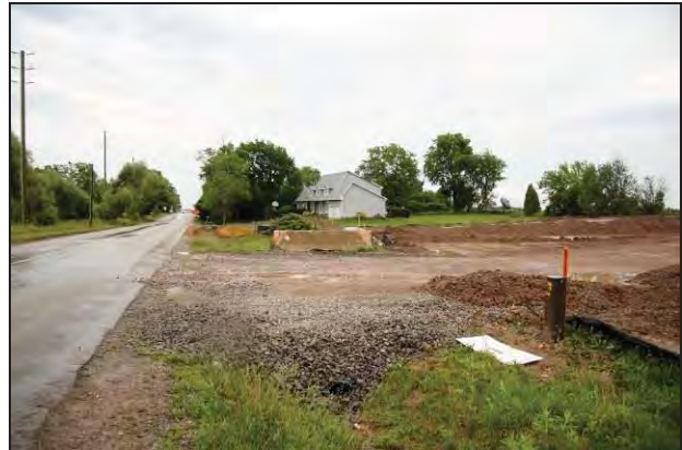
Plate 8: South view along west side of Sixth Line at construction entrance (assessed by D. R. Poulton Associates 2007).
