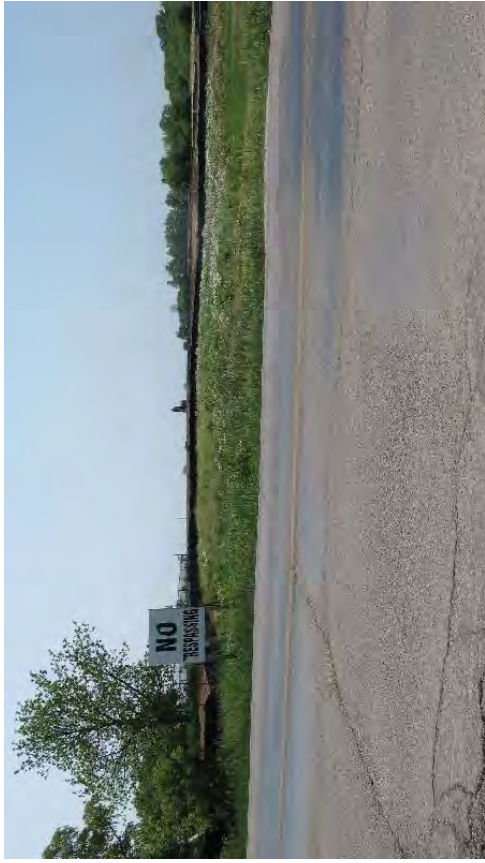
Concrete culvert northwest of Dundas Street and the current housing development on the southwest side of 6 th Line. Looking southwest.
