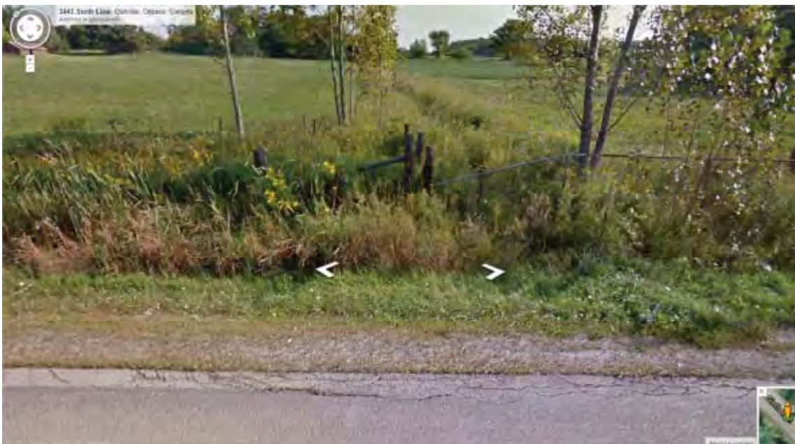
Figure 8 Looking east from Sixth Line at the ditch that inlets to culvert #4
