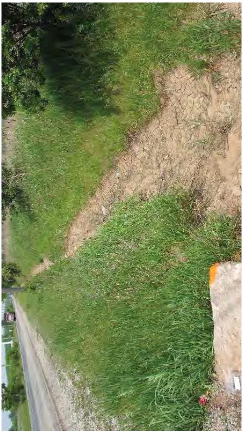
Concrete culvert northwest of Dundas Street and the current housing development on the southwest side of 6 th Line. Looking northwest.
