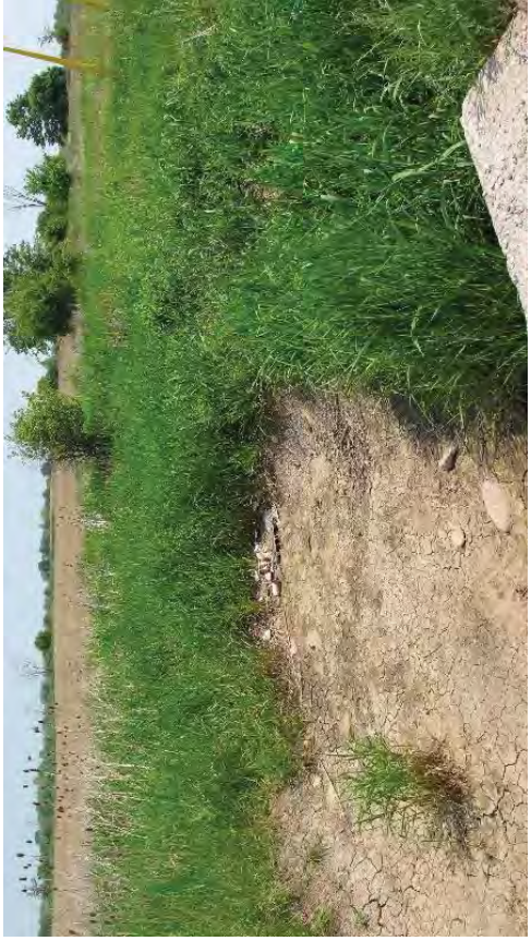
Concrete culvert northwest of Dundas Street and the current housing development on the southwest side of 6 th Line. Looking east.
