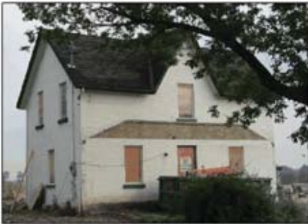
1) Boarded up windows and door openings
