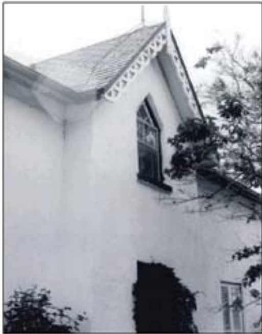
View of east elevation of the house, 1977. Photo source: Town of Oakville files
