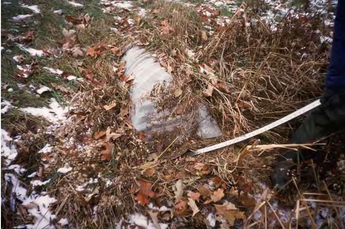
Photo 1. Reach 16WA-8 collapsed culvert.
