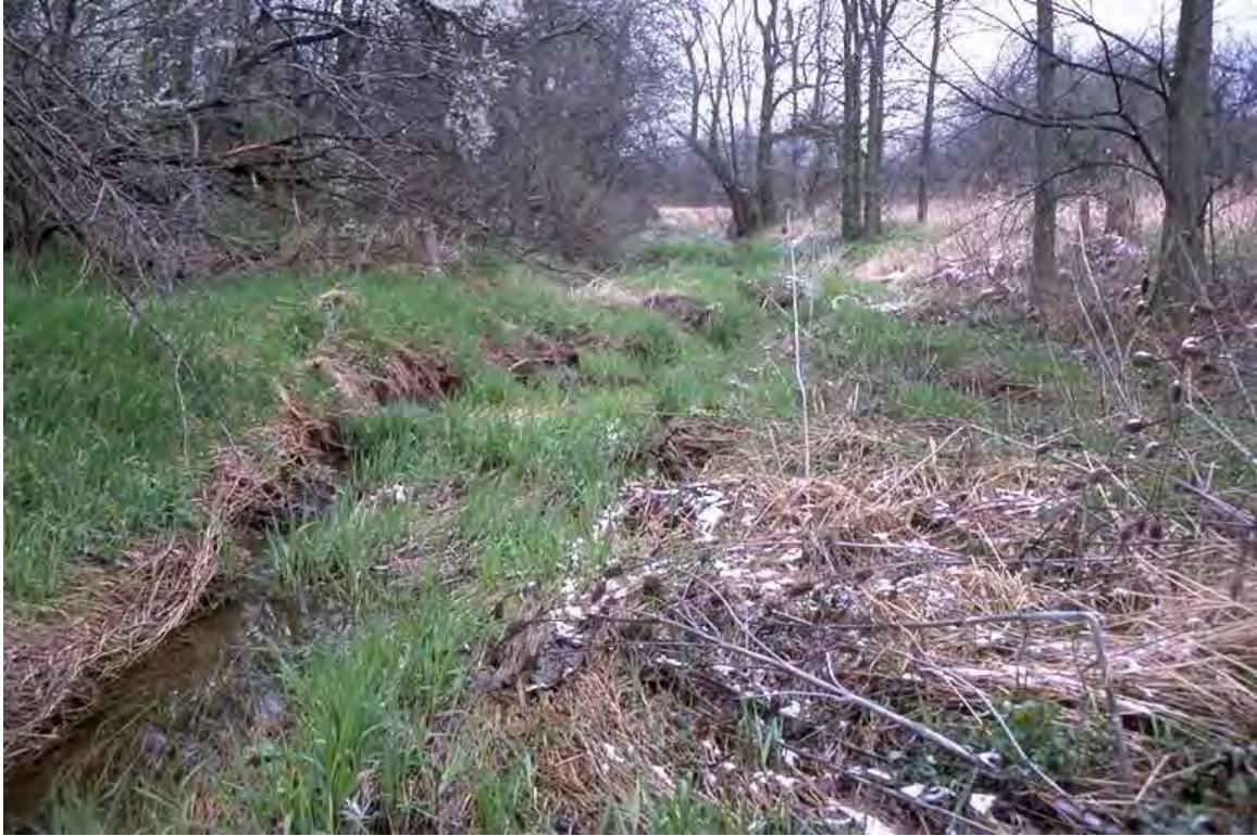
Photo 1. Reach JC-13 with slumping banks.
