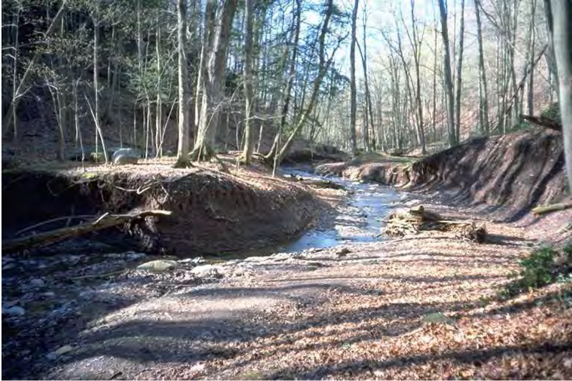
Photo 1. Reach SMA-1 bank erosion.
