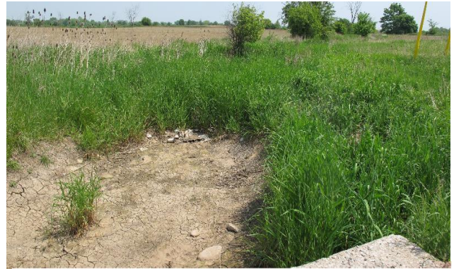
Figure 3-6 Concrete culvert northwest of Dundas Street and the current housing development on the southwest side of 6 th Line. Looking east.
