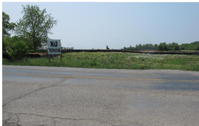
Figure 3-9 Concrete culvert northwest of Dundas Street and the current housing development on the southwest side of 6 th Line. Looking southwest.
