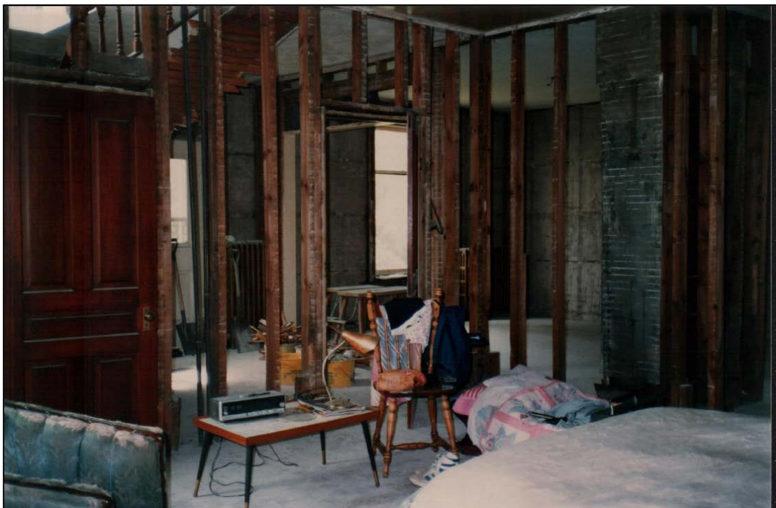
Figure 46: Interior renovation of the main level showing the exposed lath and plaster (C. Schulz, 2016).
