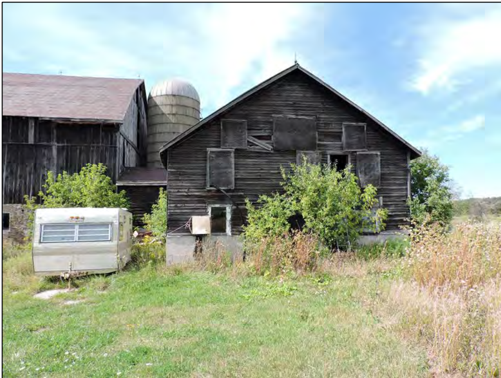
Figure 17: Small barn located at the south-east corner of the bank barn, south façade (AB, 2016).
