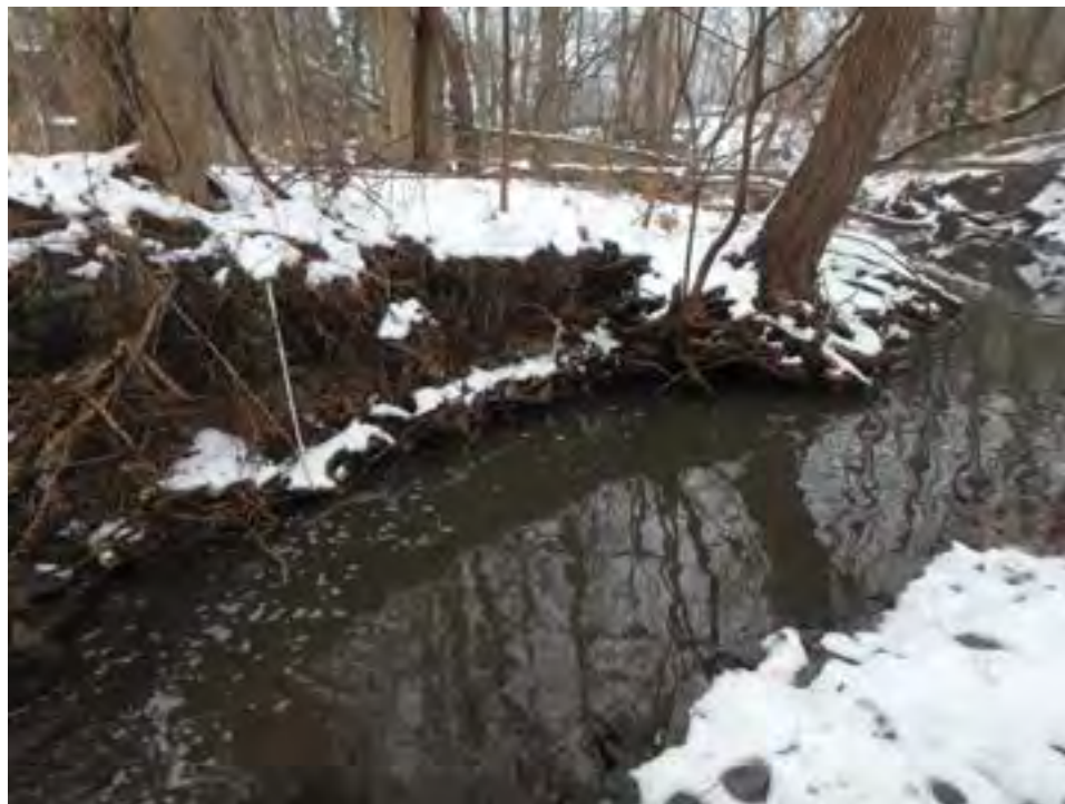
Photo 6: Erosion evident at east bank immediately downstream of Rebecca Street retaining wall.
