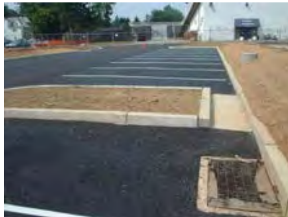
Figure 5.9 Permeable Pavement (Low Impact Development Stormwater Management Planning and Design Guide, Version 1.0, CVC and TRCA, 2010)
