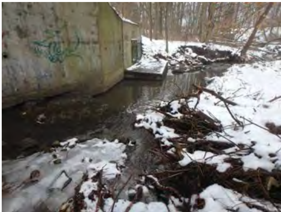
Photo 2: Cement slab present at downstream end of Rebecca Street crossing is a barrier to small-bodied fish.
