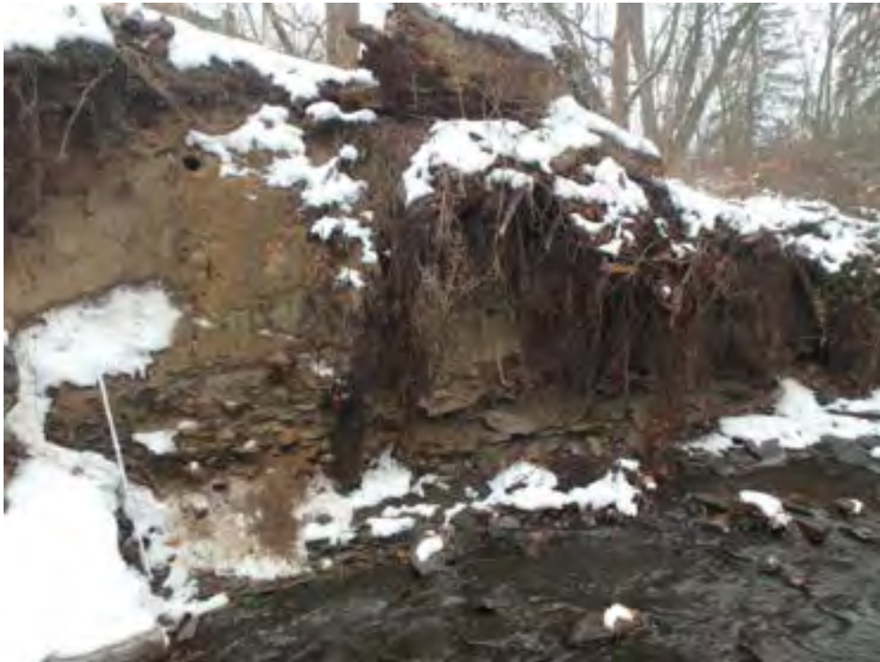
Photo 11: Bank nearest the retaining wall structure experiencing significant erosion. Erosion of bank reaches approximately 2.5 meters in height at its highest point.
