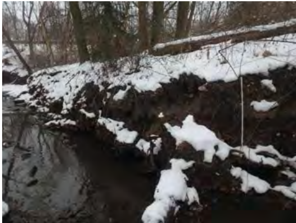
Photo 8: Erosion evident on west bank for approximately 31.5 meters prior to reaching retaining wall for Lakeshore Road.
