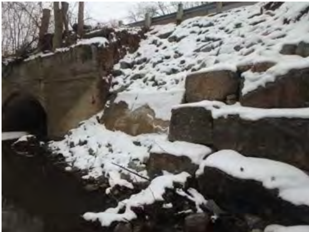
Photo 12: Emergency works were completed in the summer of 2017 to repair the severely eroded bank present directly west of the Lakeshore Road crossing.
