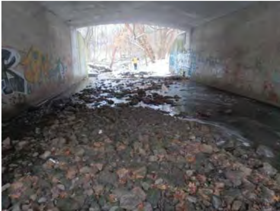
Photo 1: Within Rebecca Street ROW facing downstream. Note large area of debris at west downstream end of crossing forcing flows to move over cement ledge on east.
