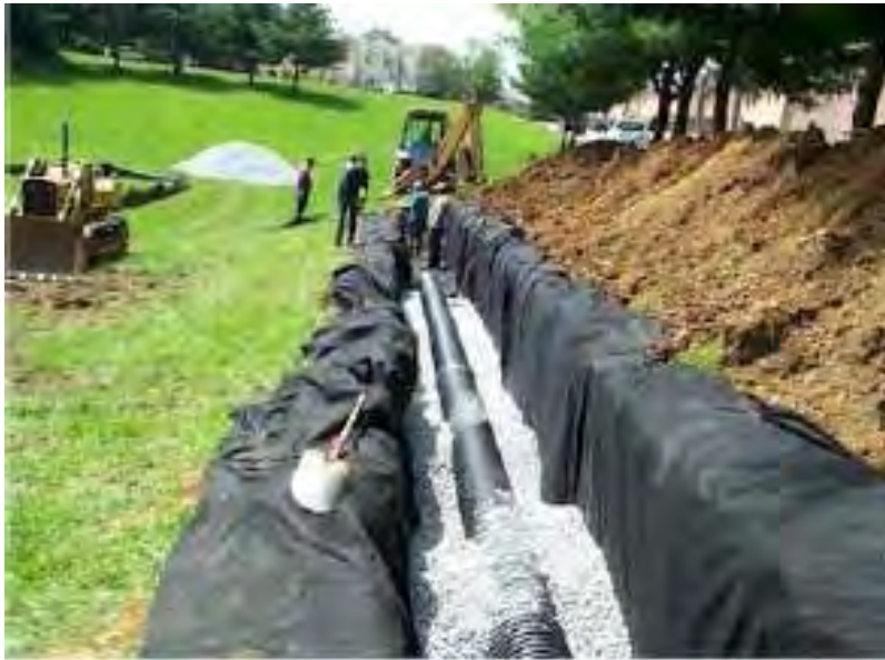
Figure 5.5 Infiltration Trench Construction (Low Impact Development Stormwater Management Planning and Design Guide, Version 1.0, CVC and TRCA, 2010)
