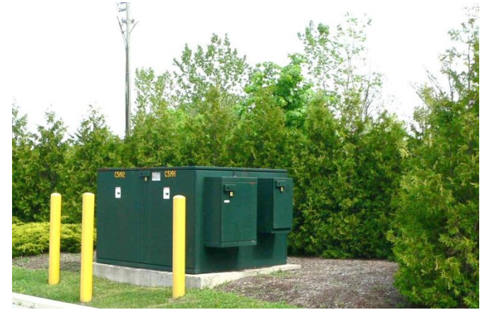
Plant material screens transformer while not interfering with access or maintenance (2.2.15)
