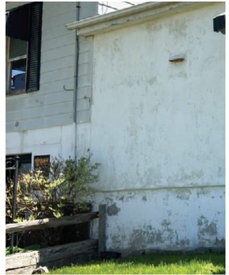
Concrete block wall mostly in fair condition despite defects (ERA, 2025).
