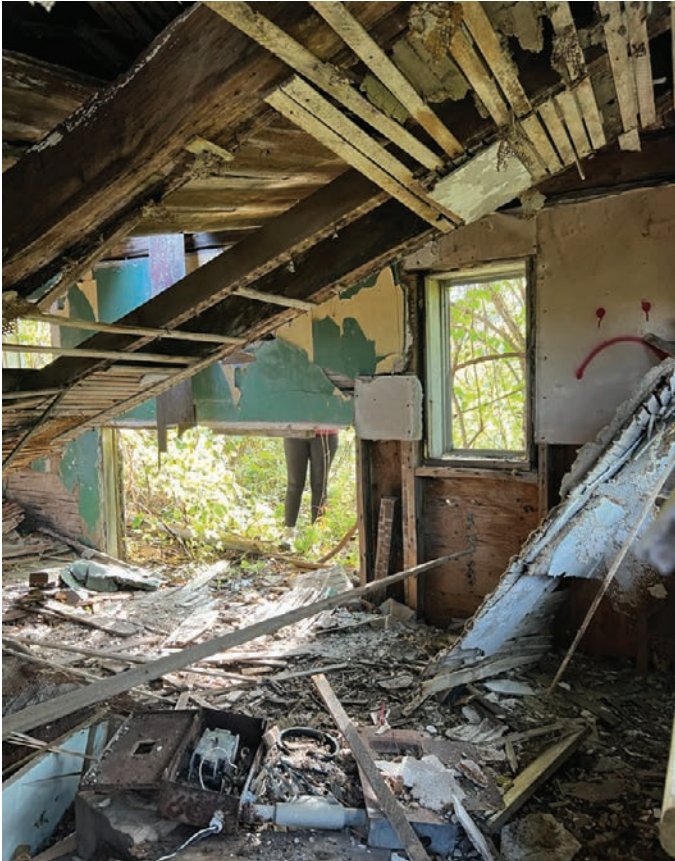
Collapsed second storey and large opening at side (south) elevation (ERA, 2025).
