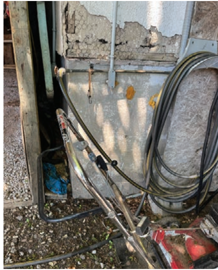
Stucco in poor condition, showing delamination (ERA, 2025).
