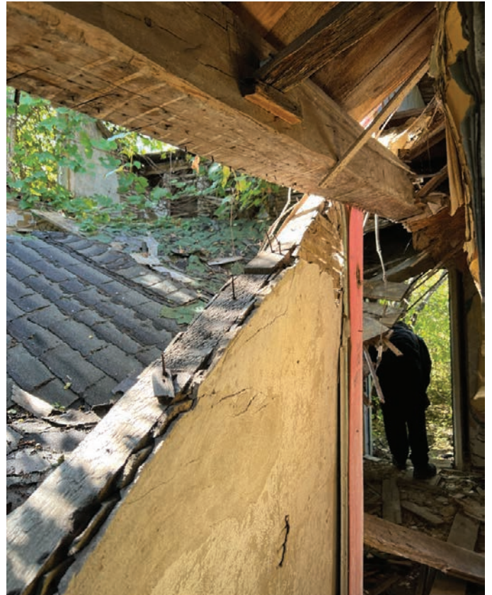
Collapsed floor on the south side of the house. Note the hewn timber beam (ERA, 2025).
