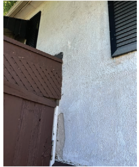
Stucco in poor condition, showing cracking and delamination (ERA, 2025).
