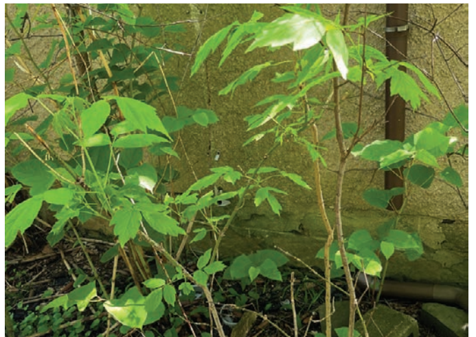
Missing downspout section near the foundation (ERA, 2025).
