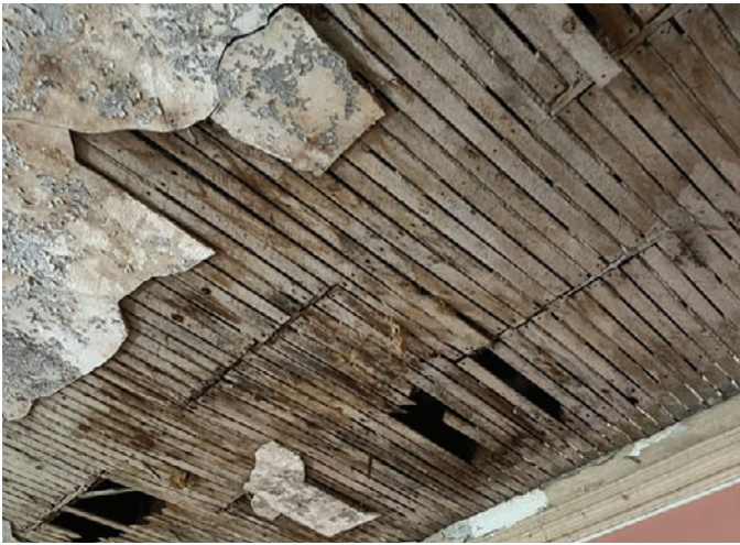
Plaster ceiling at original portion of building in poor to defective condition, showing large areas of missing material (ERA, 2025).
