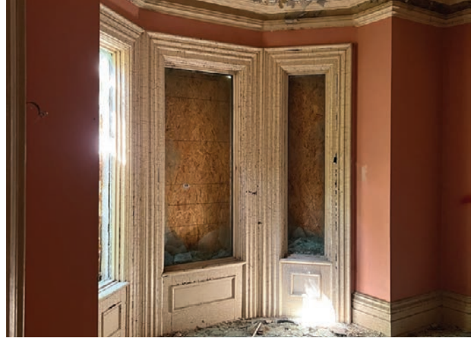
Window surrounds in fair condition (ERA, 2025).
