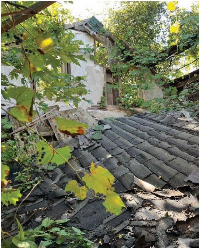
Collapsed roof and exposed gable end (ERA, 2025).
