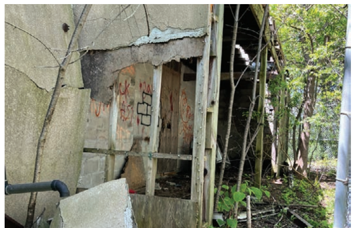
Concrete block wall in fair condition, with sections of graffiti (ERA, 2025).
