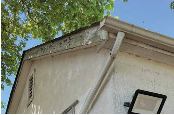
Bargeboard, fascia and soffit show paint flaking, wood rot and cracking (ERA, 2025).
