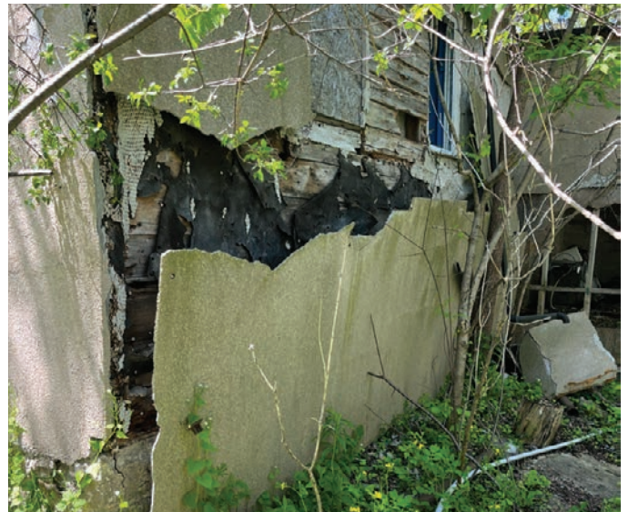
Areas of stucco in defective condition (ERA, 2025).
