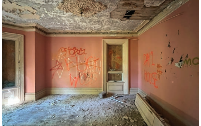
Interior spaces generally in defective condition (ERA, 2025).
