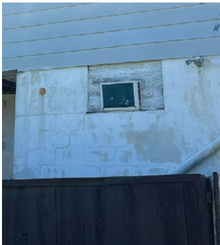
Concrete block wall with areas of poor condition, including step cracking (ERA, 2025).
