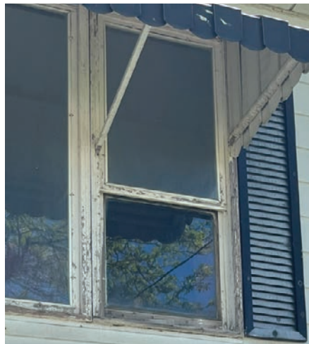
Wood windows in poor condition, with areas of wood rot (ERA, 2025).
