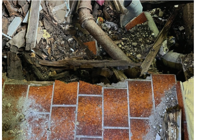
Tile floors at the later addition in defective condition (ERA, 2025).
