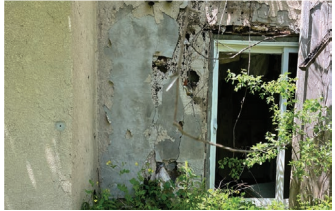
Stucco facade at the side (south) elevation in poor condition (ERA, 2025).
