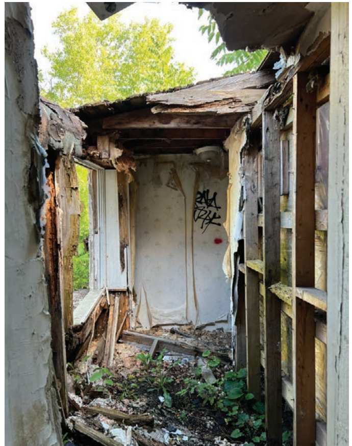
The roof in the 20th-century two-storey addition has failed (ERA, 2025).
