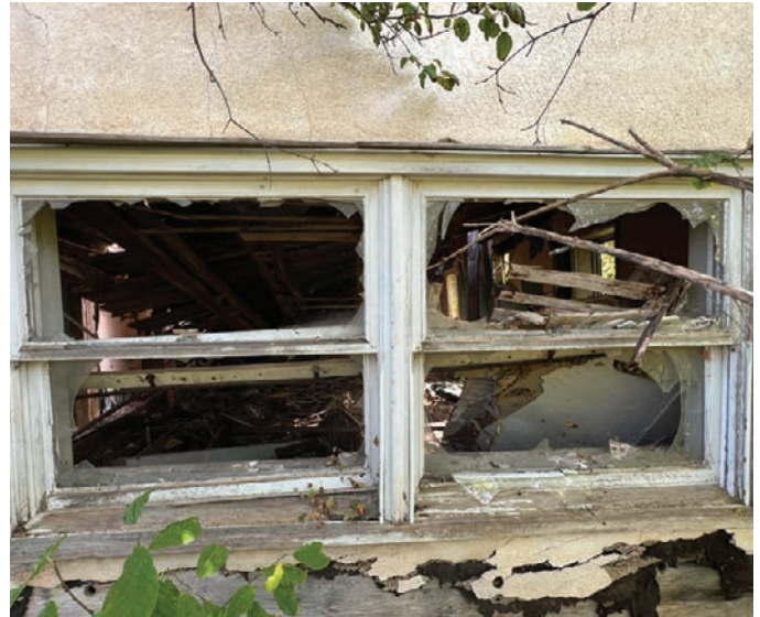
Close-up photo of window on principal (west) elevation in defective condition, with missing glazing (ERA, 2025).
