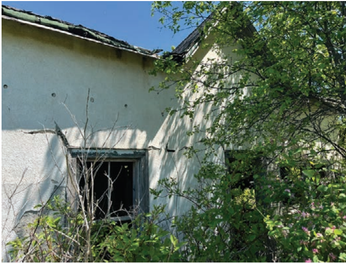
Dense vegetation at the principal (west) elevation (ERA, 2025).
