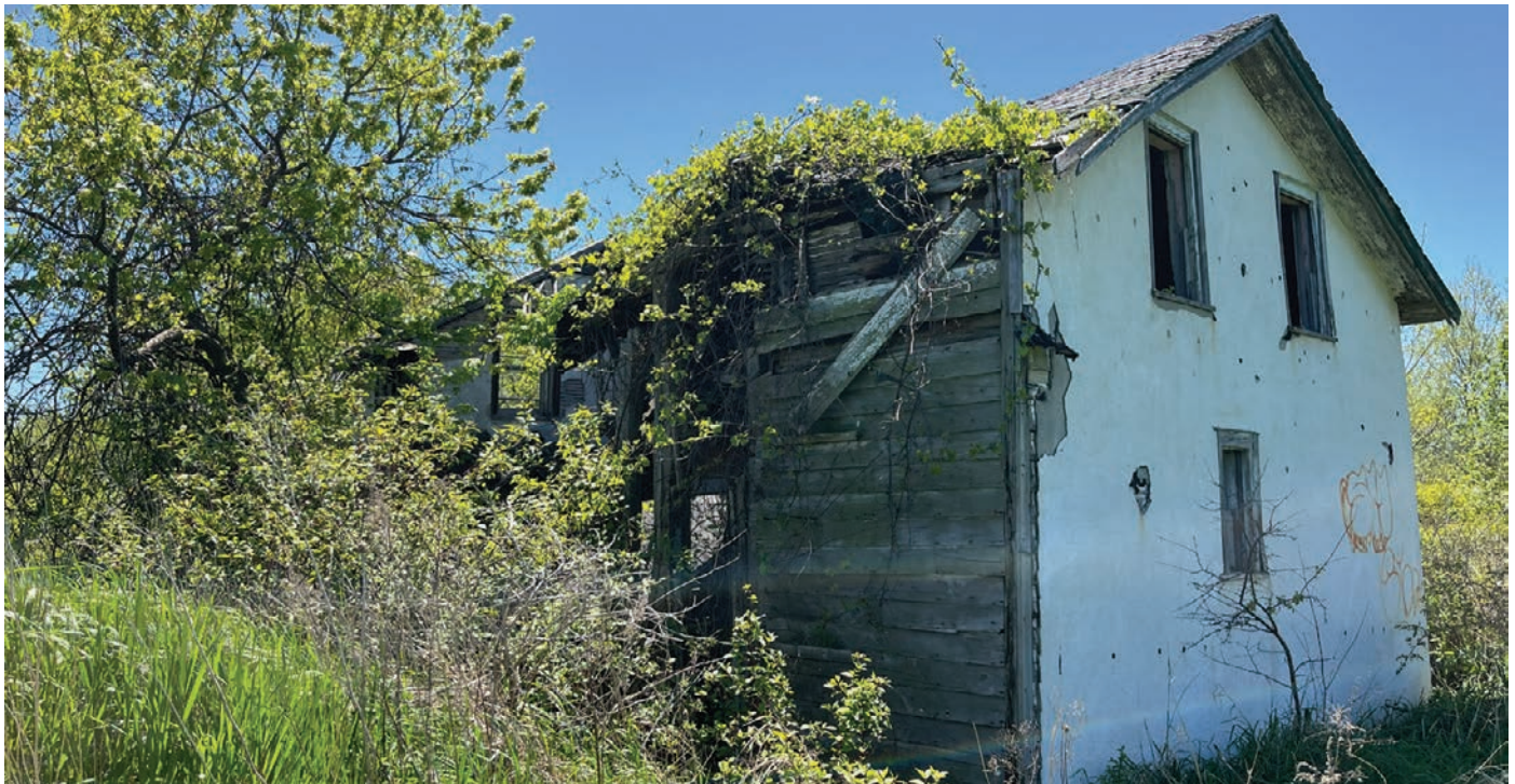
Side (south) and rear (east) elevations of the circa 1840s building at 340 Burnhamthorpe Road. Note the failure and collapse of the rear wall (ERA, 2025).
