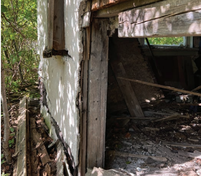
Large opening on the south elevation where a fireplace would likely have been located (ERA, 2025).
