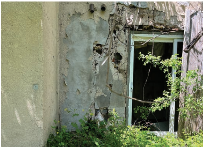
Sliding door on side (south) elevation in defective condition (ERA, 2025).
