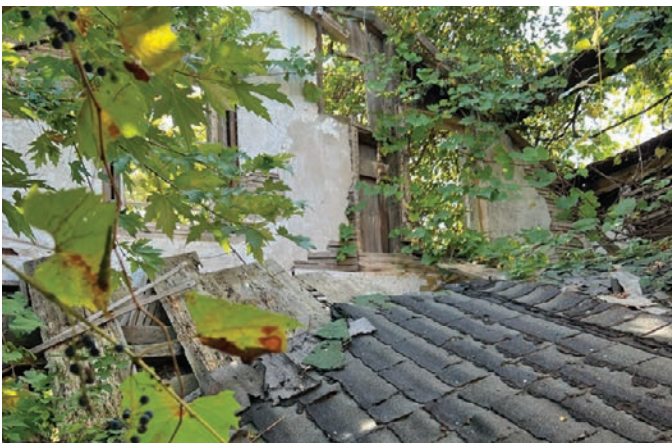
Partially collapsed roof and missing framing have exposed part of the second storey to the elements (ERA, 2025).
