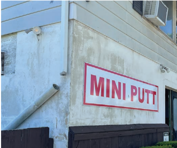
Metal eavestrough and downspouts in fair condition with an area of poor condition, with a missing downspout elbow (ERA, 2025).
