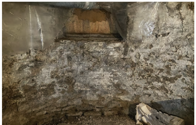
Fieldstone foundations, viewed from the basement, in poor condition (ERA, 2025).
