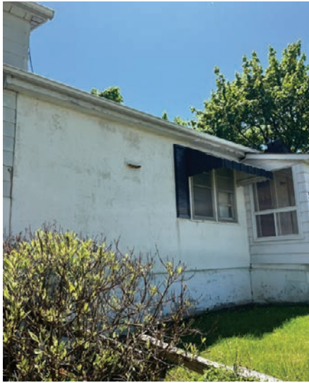
Stucco in poor condition (ERA, 2025).
