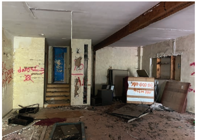
Ceiling at the north part of the later addition in poor condition (ERA, 2025).
