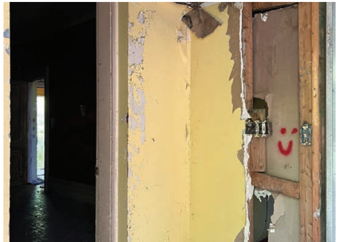
Drywall at the later addition in poor to defective condition (ERA, 2025).
