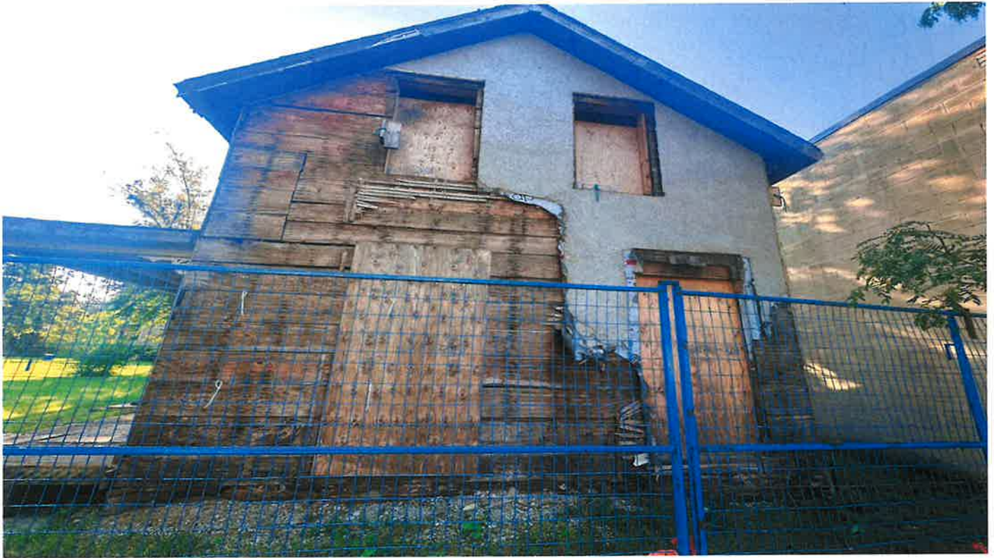
General view of west house located at the subject site (looking South)
