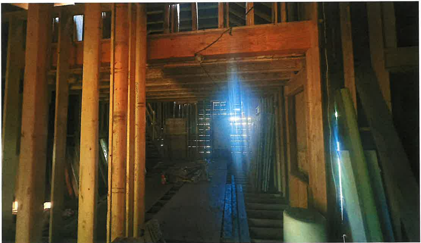
General view of the house located at the western portion of the subject site (looking North)
