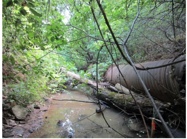
Photo <6>. View of old culvert downstream of golf cart path in Tributary 14W-W1 (Aug, 2012).
