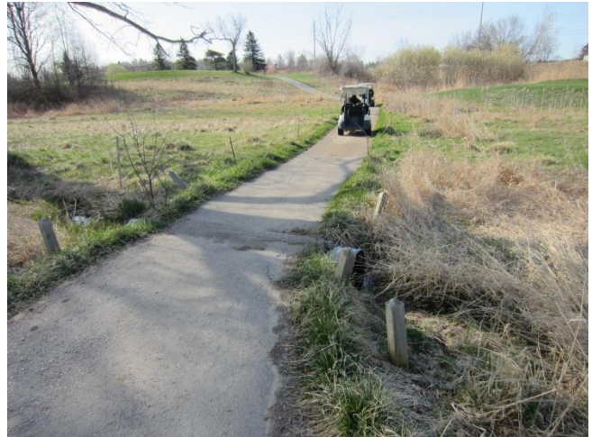
Photo <4>. View of culvert along golf cart path downstream of confluence 14W-W1-2 and 14W-W1-3 (March, 2012).
