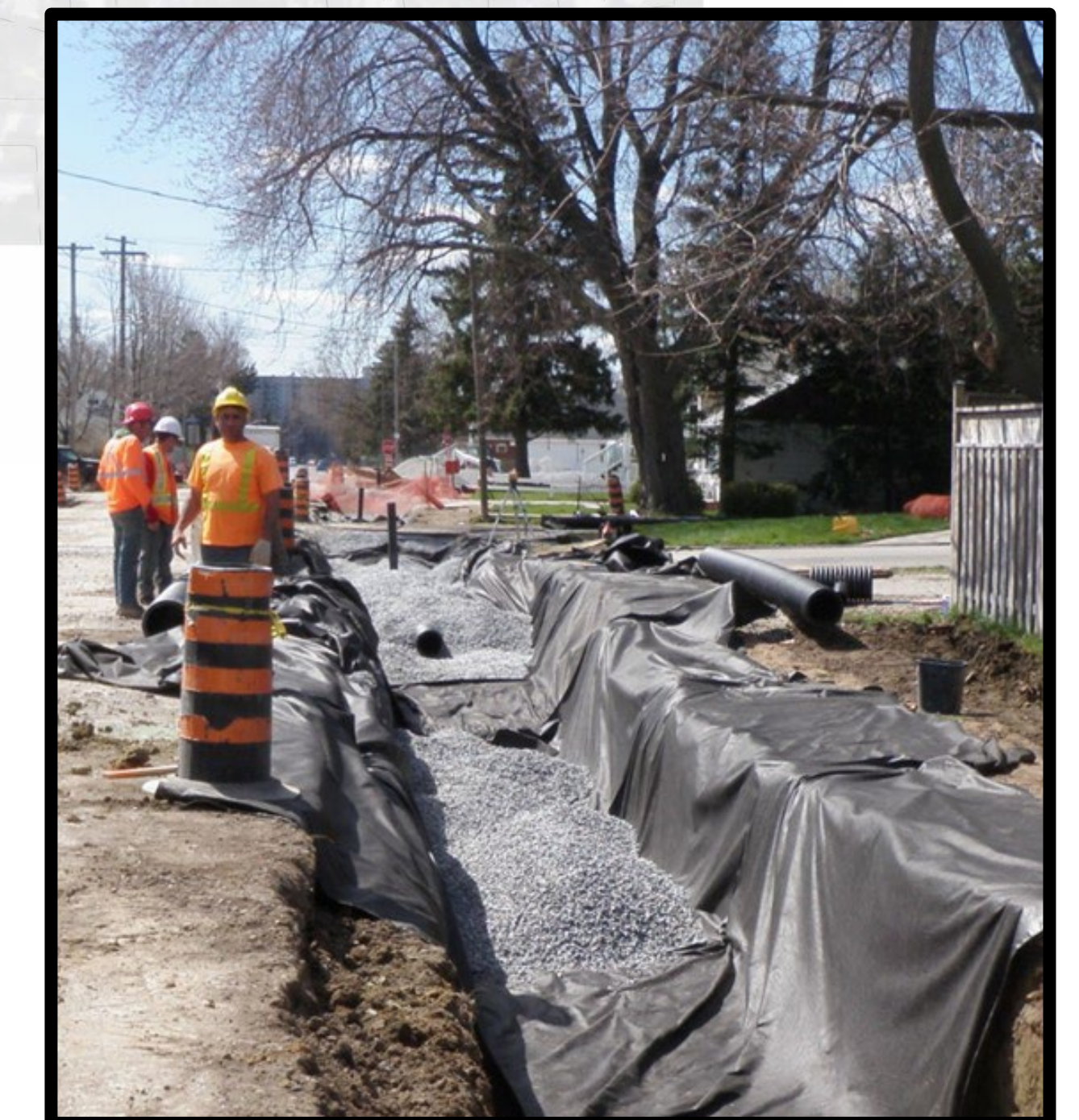
Alt 4B: LID/ Green Infrastructure enhancement (perforated pipe) to existing storm sewer upgrades and new storm sewers)
