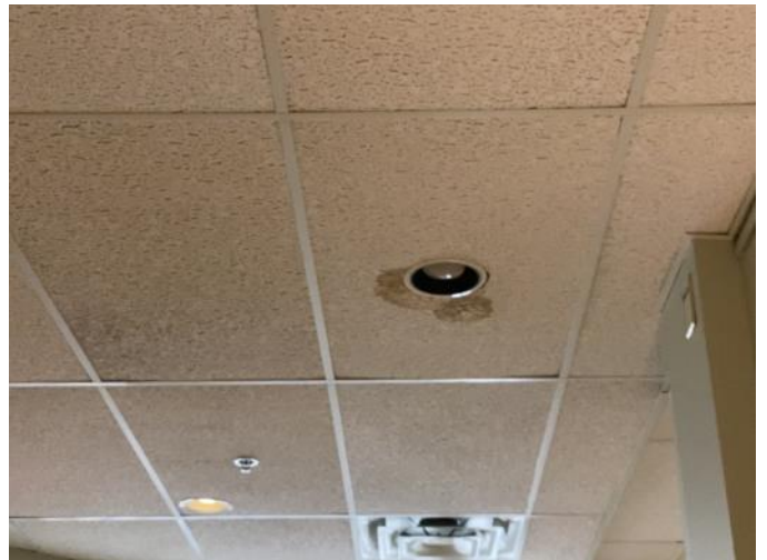
Photo 14: View of water staining observed on the ceiling tiles of the second floor (radio station unit).
