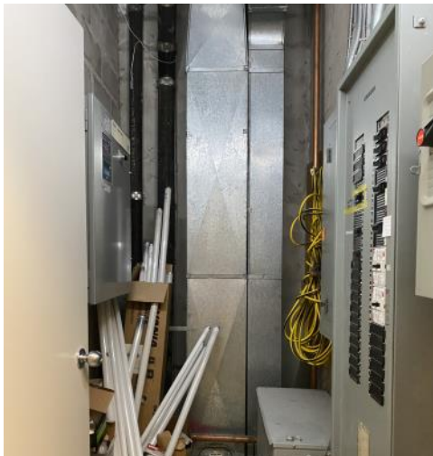
Photo 13: View of the utility room on the second floor (radio station unit)
