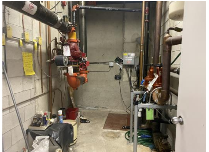
Photo 8: View of the basement plumbing utility room, where the sump pump was located.
