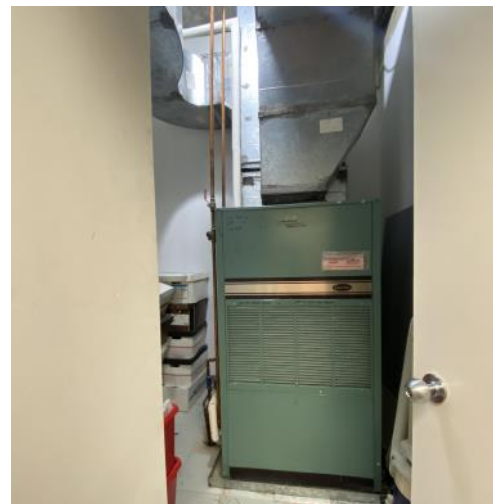
Photo 12: View of the air handler in the radio station unit (second floor).
