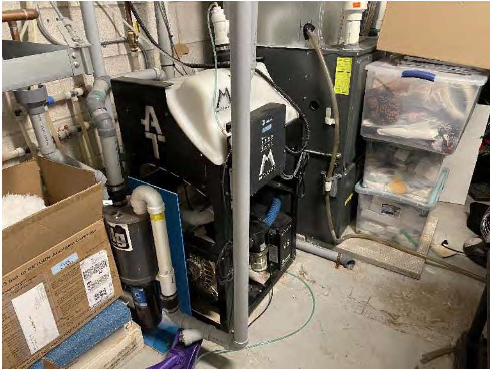
Photo 9: Disinfection system for the dental office at 165 Cross Avenue.
