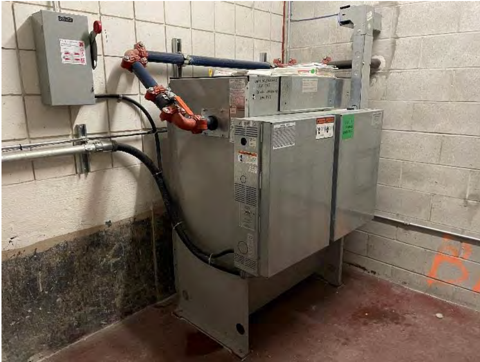
Photo 5: The hydraulic oil AST at the back of the Site building at 165 Cross Avenue, used for the elevator, no leaks have been reported.
