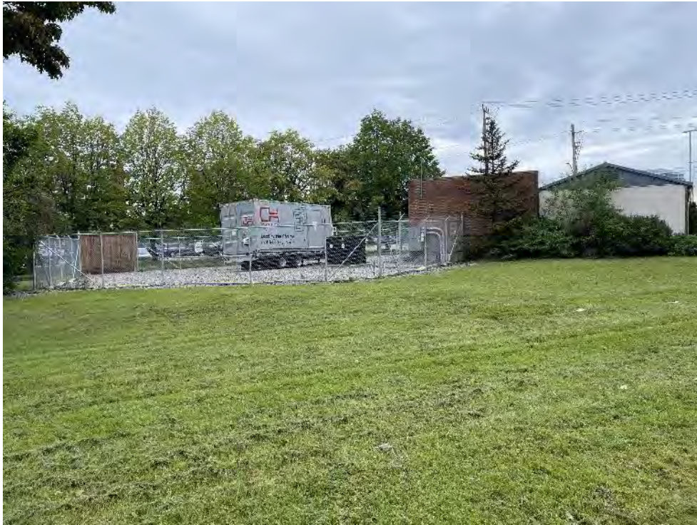
Photo 19: The property located at 539 Lyons Lane, approximately 150 m southwest, is occupied by a power station with a transformer.
