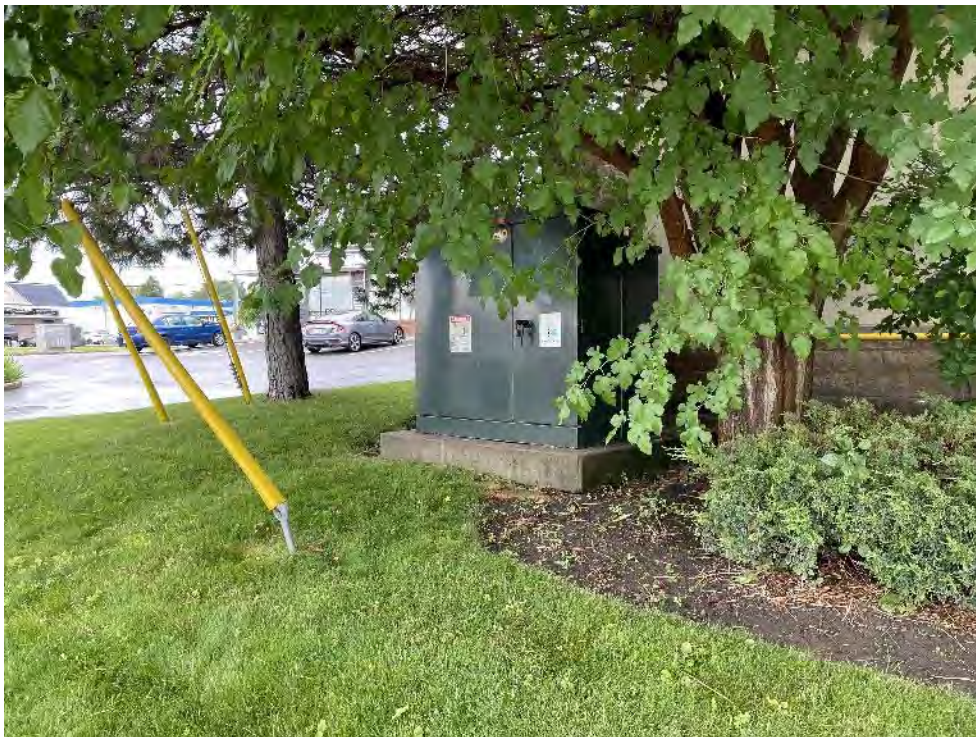
Photo 18: One (1) transformer was observed at the property located at 217 Cross Avenue, approximately 140 m northeast. Based on the label, it was manufactured in 2003, which is unlikely to contain PCBs.
