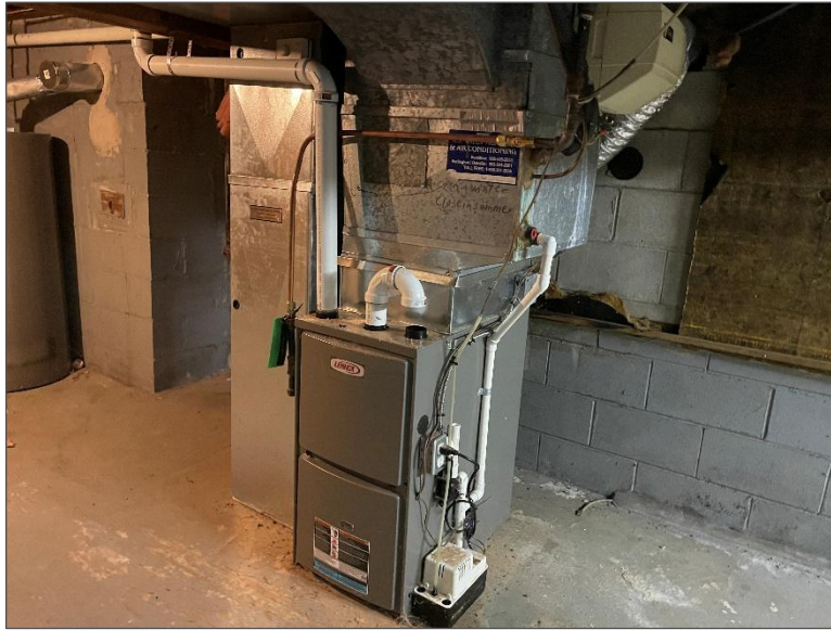
Photograph 11 – Air-forced furnace located in the basement of the Site Building.
