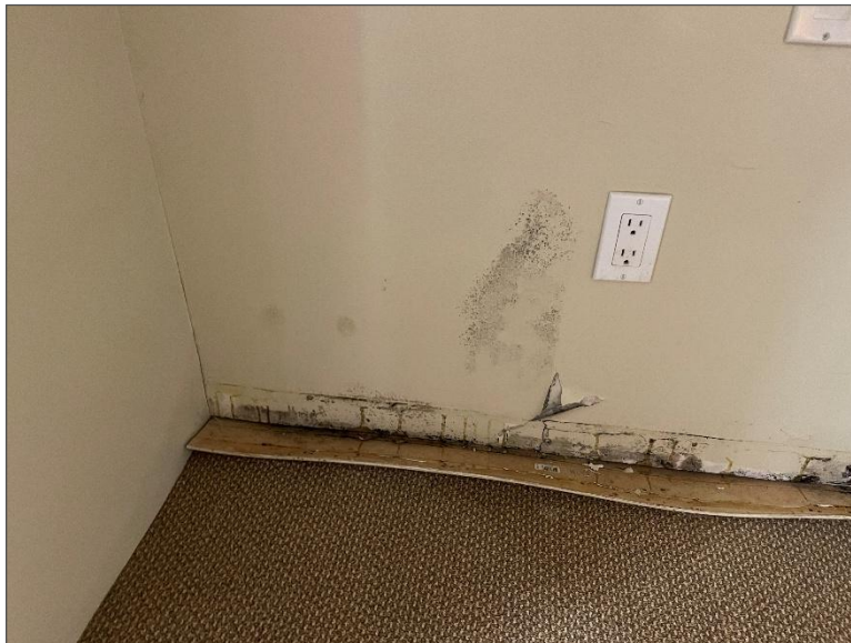
Photograph 12 – Suspect mould growth observed in the basement of the Site Building.
