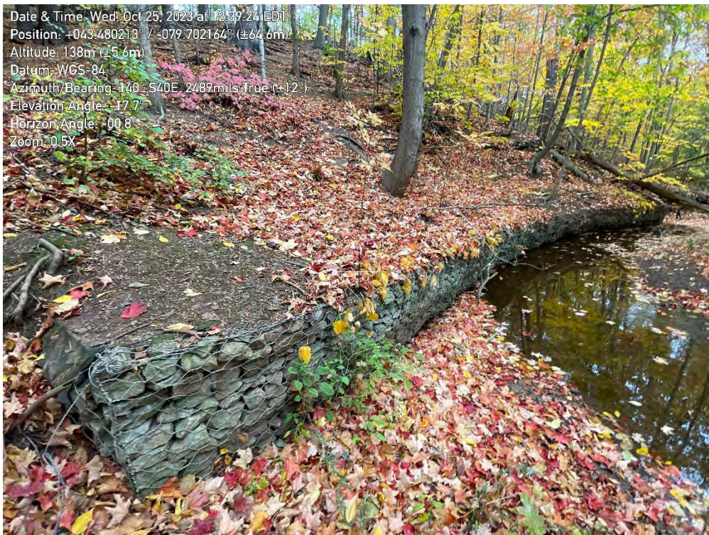
Photo 4. View of undercut gabion baskets in Zone B17 of the East Morrison Creek, looking Southeast.
