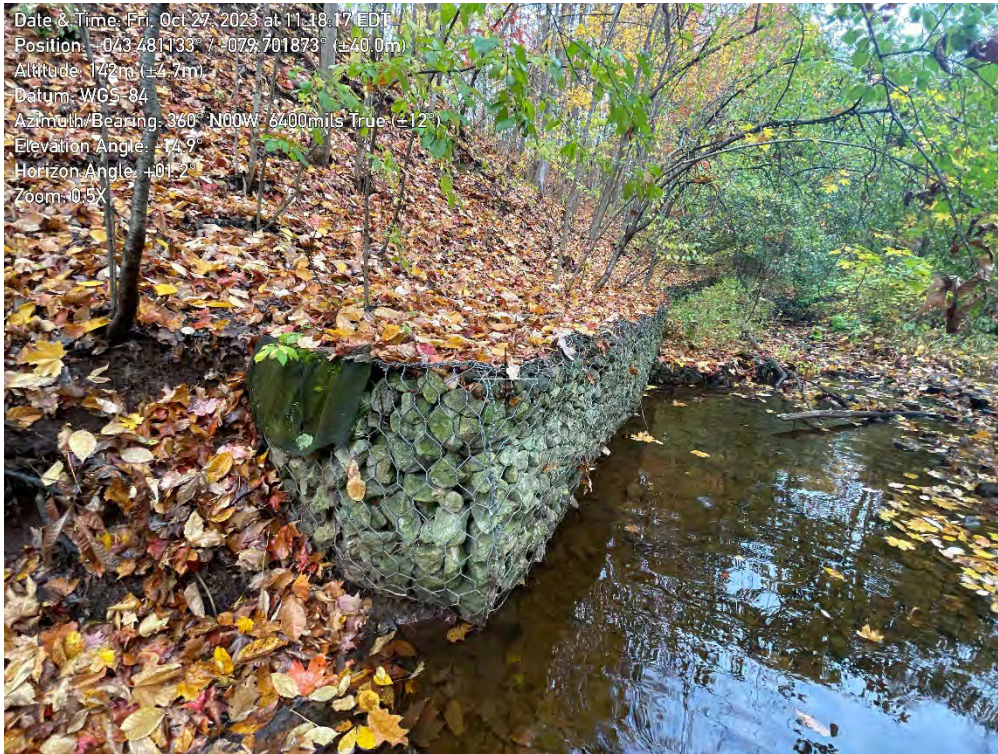
Photo 3. View of undercut gabion baskets in Zone A19-2 of the East Morrison Creek, looking Northwest.
