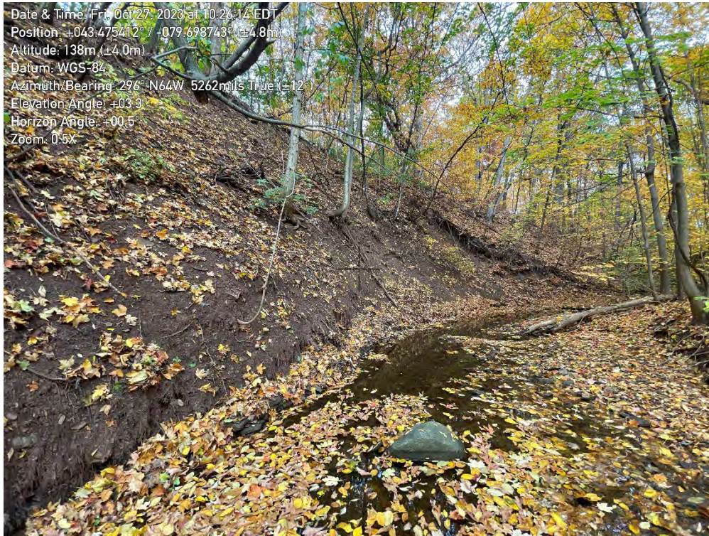
Photo 27. View of erosion in Zone A13 of the East Morrison Creek, looking Northwest.
