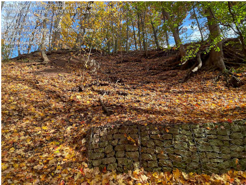
Photo 42. View of valley wall slope in Zone B32 of the East Morrison Creek, looking Northeast.
