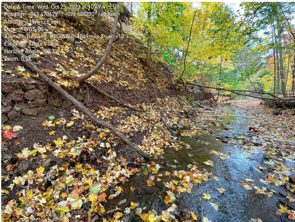
Photo 166. View of the buried gabion baskets in Zone B2 of the East Morrison Creek, looking Southeast.
