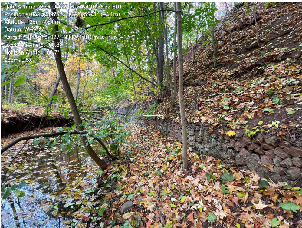
Photo 2. View of failed gabion baskets in Zone B13 of the East Morrison Creek, looking Northwest.
