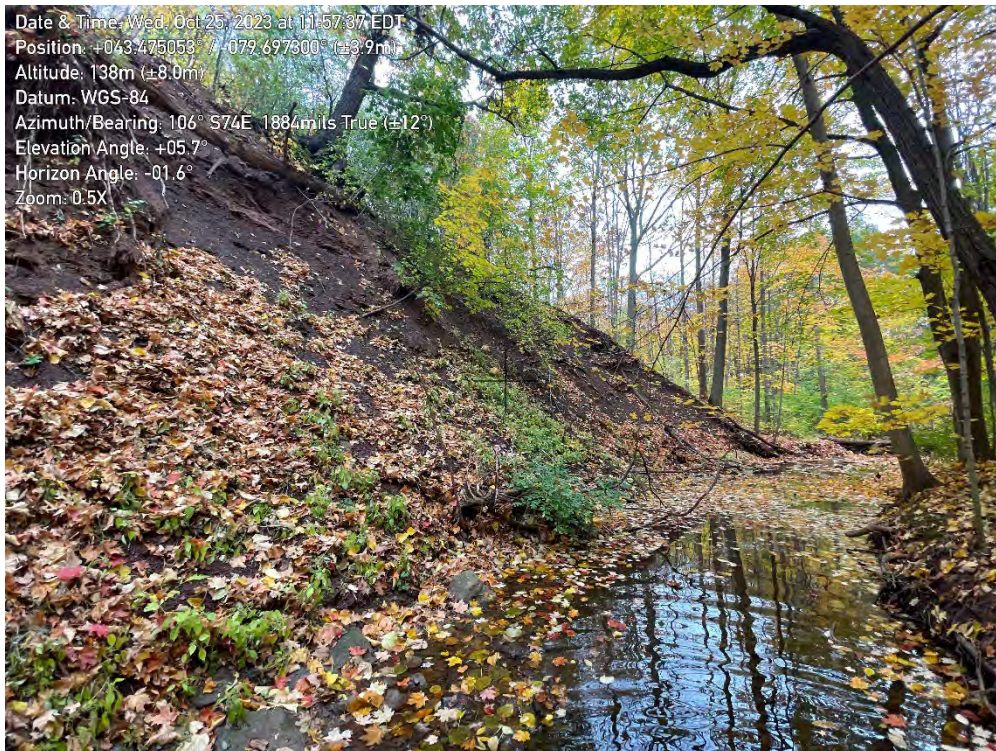
Photo 40. View of erosion in Zone B11 of the East Morrison Creek, looking Southeast.
