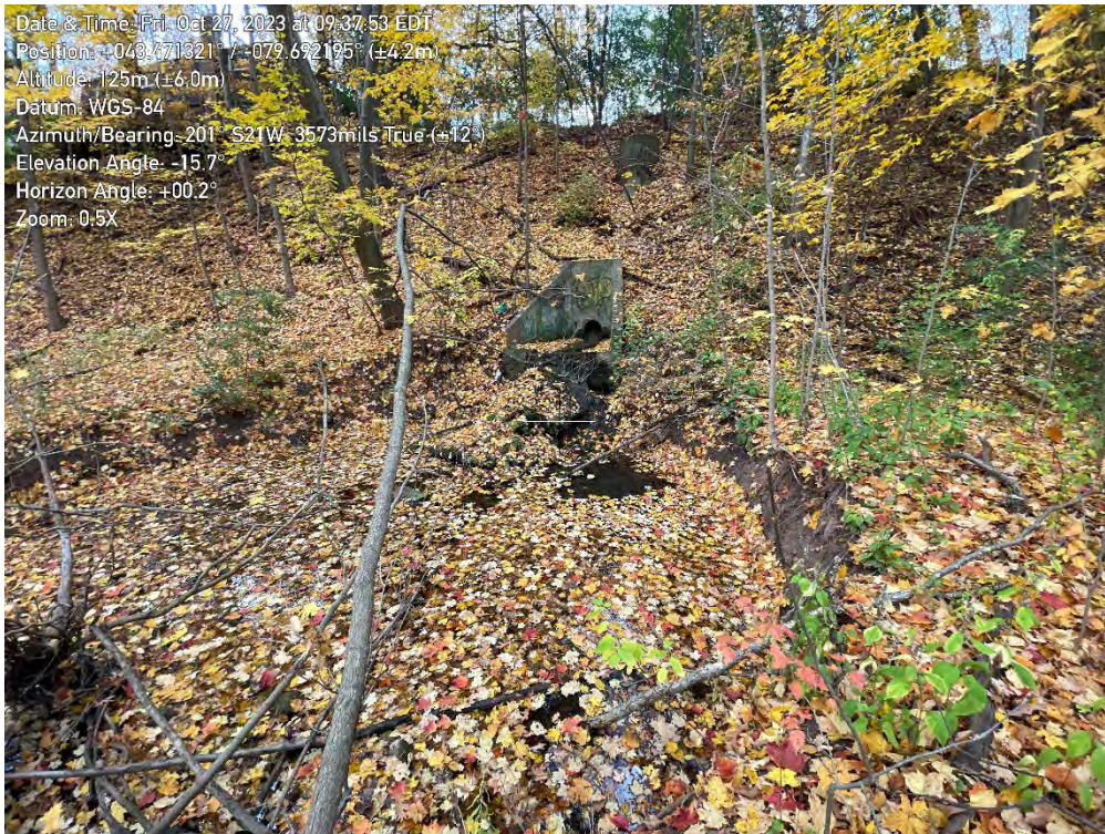
Photo 6. View of failed outflow culvert in Zone A7 of the East Morrison Creek, looking Southwest.
