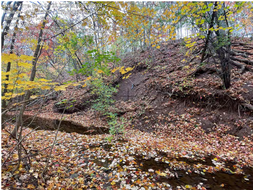
Photo 38. View of erosion in Zone B9 of the East Morrison Creek, looking Northeast.
