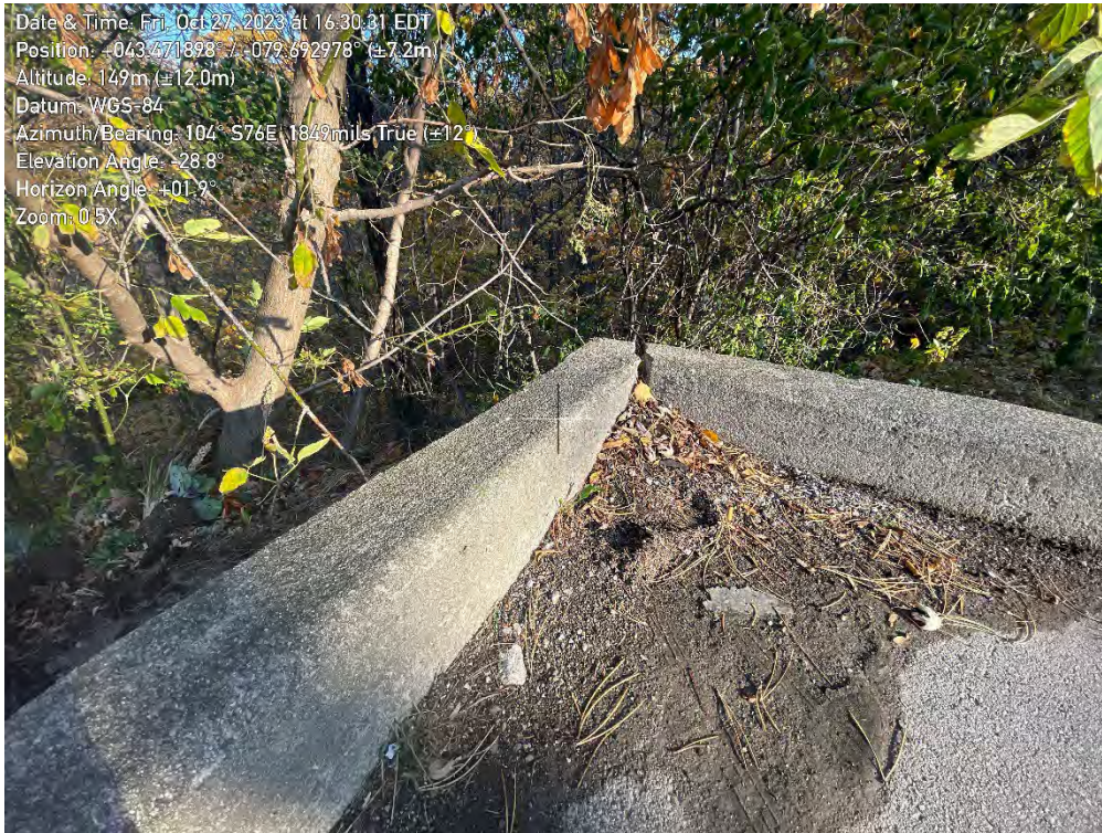
Photo 11. View of separating parking lot curbs at 1359 White Oaks Boulevard, slope crest of Zone A7, looking Southeast.
