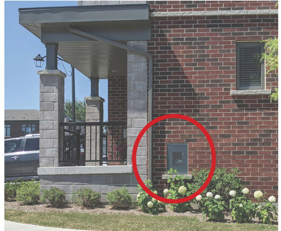
Fig. 7.6 - Utilities should be discreetly located, integrated into the architecture or screened from public view
