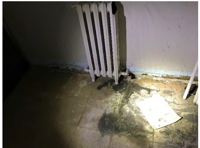
Photo 12: Evidence of black staining surrounding a radiator in the basement
