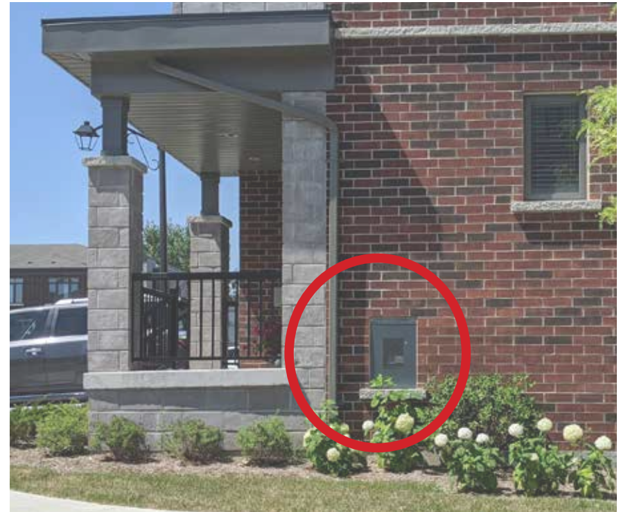
Fig. 6.5.6a - Utilities should be discreetly located, integrated into the architecture or screened from public view
