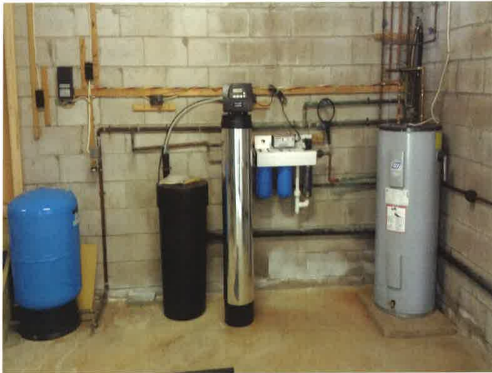
View of water filtration unit in the basement of Residence A
