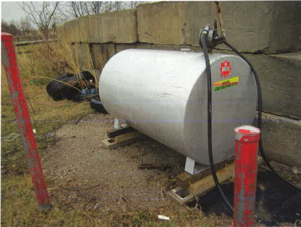
General view of an AST at north of the stable (facing northeast)
