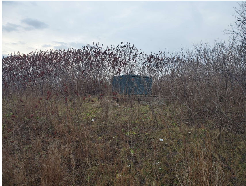
Photo 11 View of termination compartment and vault, southeast adjacent to Site, facing southwest
