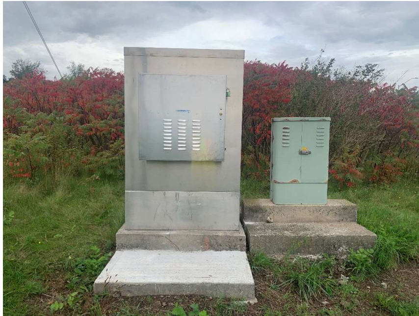
Photo 7 View of two traffic signal switch boxes south adjacent to Site, facing north
