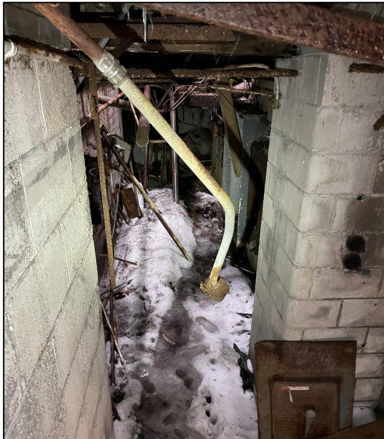
Photograph 4: Condition of basement observed from grade (March 2025 Assessment)
