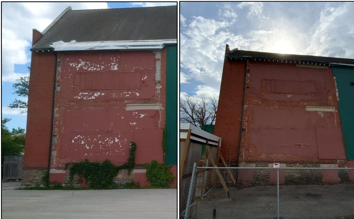
Photograph 18: North elevation flashing failure (2016 – Left, March 2025 – Right)
