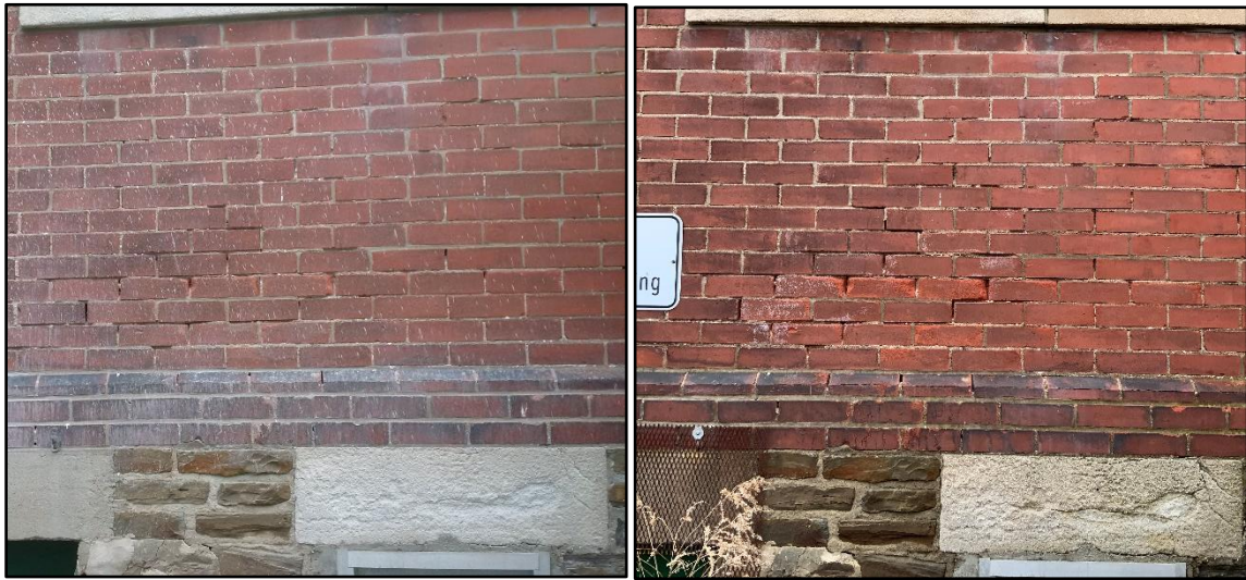
Photograph 19: East elevation brick spalling and mortar loss (2016 – Left, March 2025 – Right)
