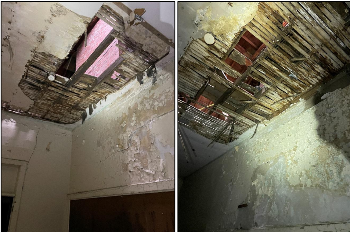
Photograph 8: Damage to ceiling framing due to open roof hatches (March 2025 Assessment)
