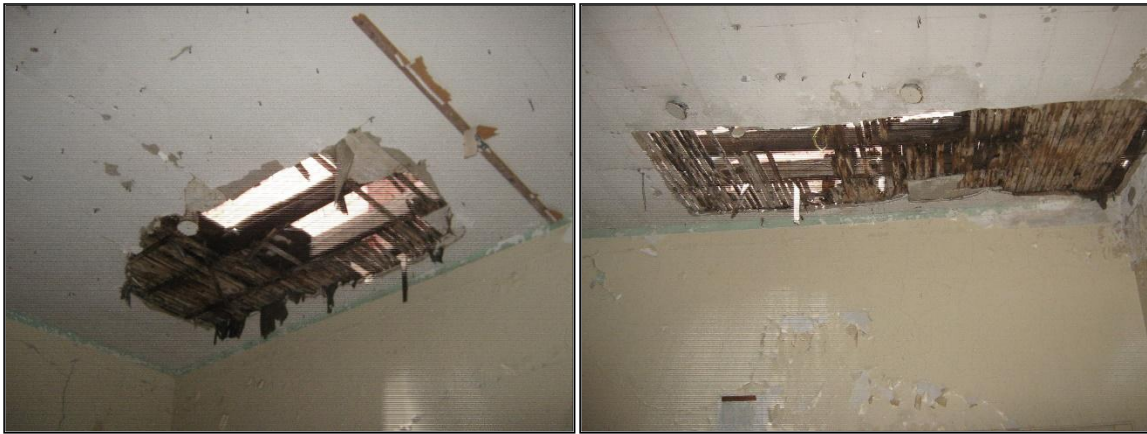
Photograph 7: Damage to ceiling framing due to open roof hatches (2016 Assessment)
