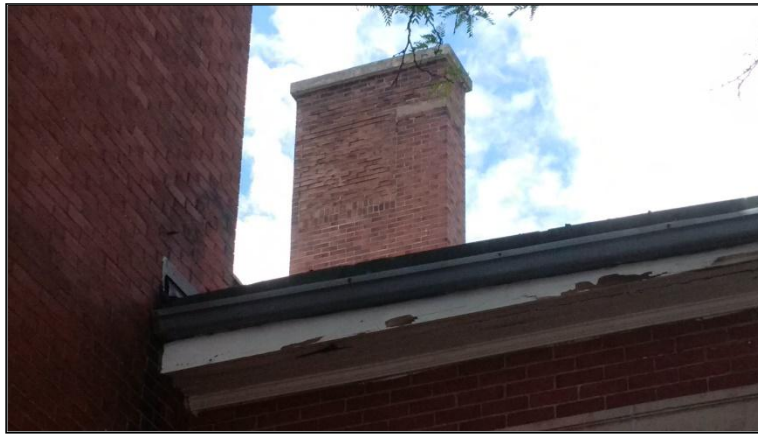
Photograph 17: Mortar loss and brick damage to chimney masonry (2016 assessment)
