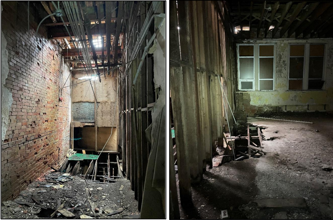
Photograph 12: Collapsed main-floor east framing (March 2025 Assessment); compare Photograph 9
