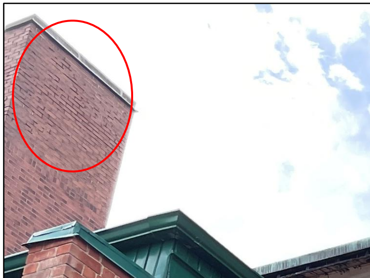
Photograph 22: Mortar loss and brick damage to chimney masonry (March 2025 assessment)
