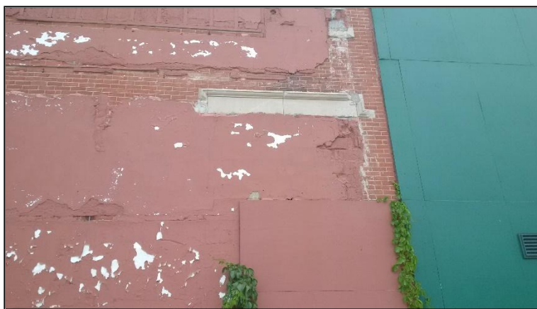
Photograph 15: Damaged decorative stone lintel (2016 Assessment)
