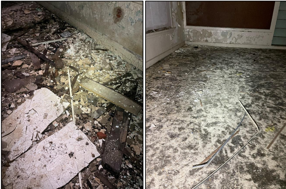
Photograph 13: Damage to second floor framing (March 2025 Assessment)
