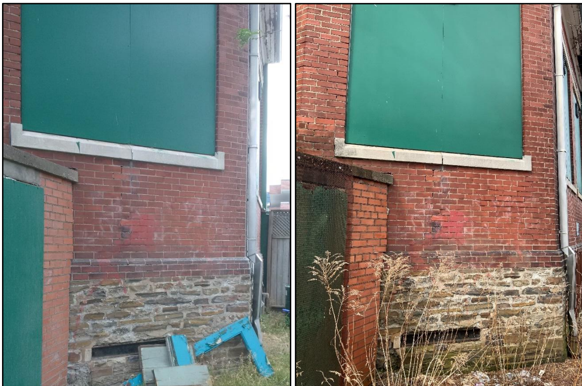
Photograph 20: East elevation brick spalling and mortar loss (2016 – Left, March 2025 – Right)
