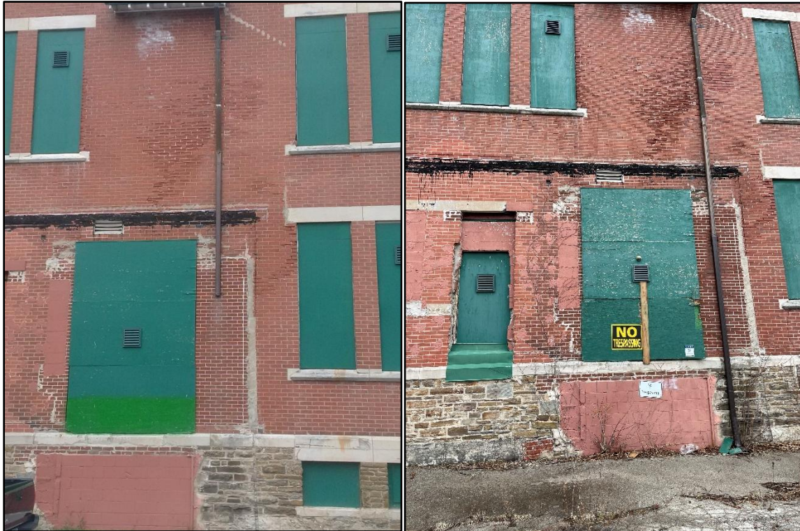
Photograph 21: West elevation brick spalling and mortar loss (2016 – Left, March 2025 – Right)
