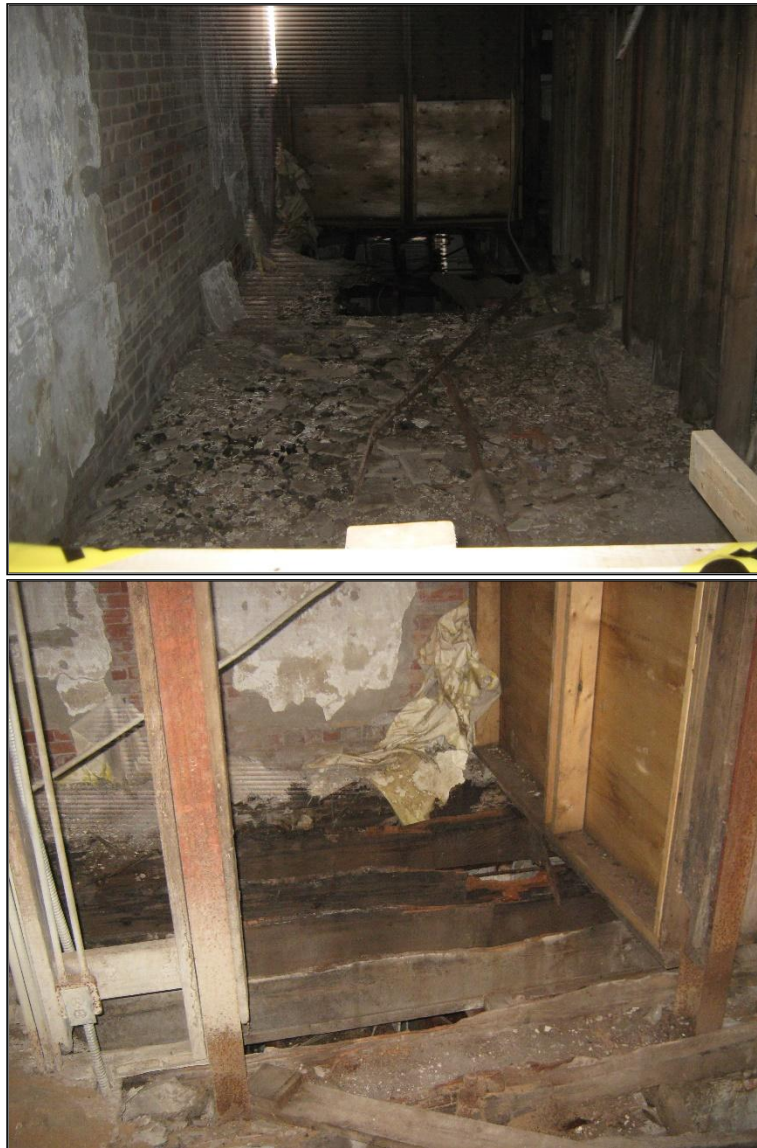
Photograph 10: Collapsed main-floor east framing (2016 Assessment)
