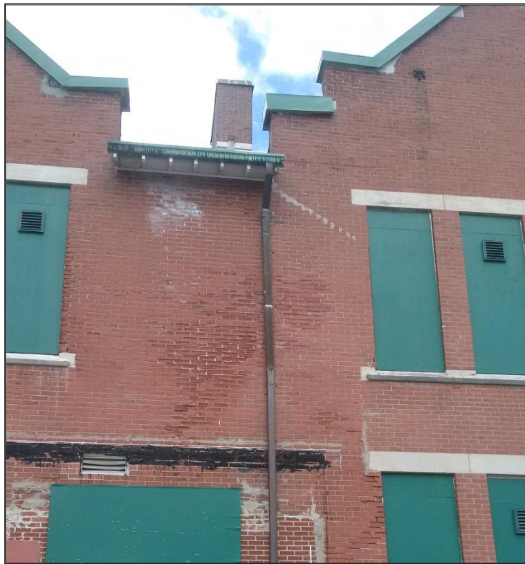
Photograph 16: Masonry spalling and mortar loss at west elevation (2016 Assessment)
