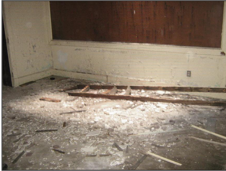
Photograph 11: Damage to second floor framing (2016 Assessment)
