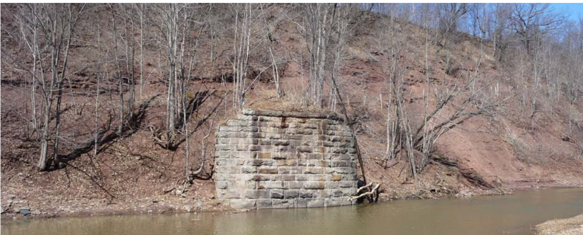
Example of a listed potential cultural heritage landscape: the Glenorchy Bridge remnants at Fourth Line.
