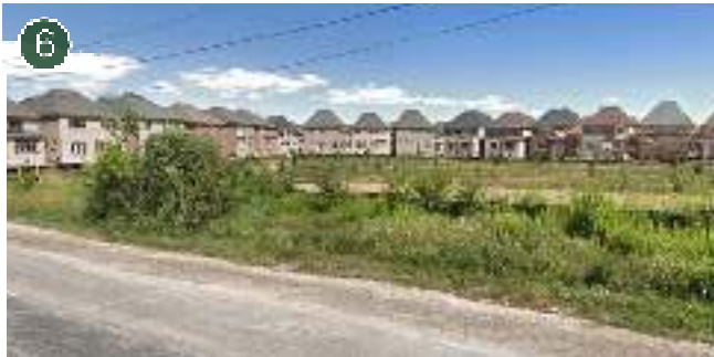
Existing single detached houses under construction backing onto NHS channel along east side of Sixth Line, south east of the Argo West Morrison Creek subject lands.
