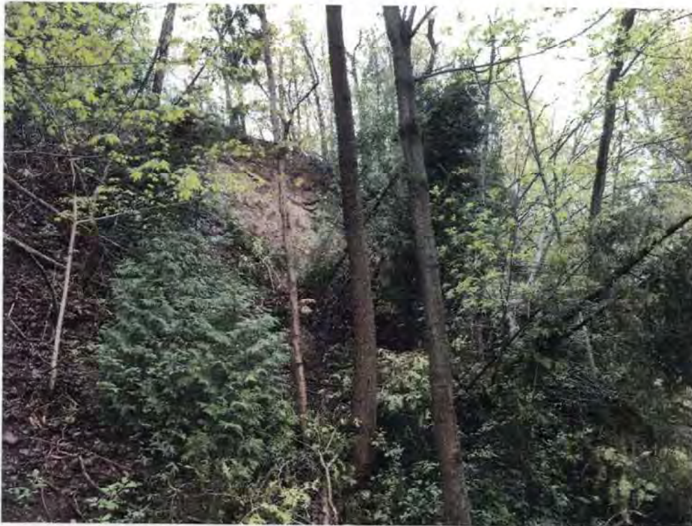
Sixteen Mile Creek Slope – Looking Northwest, slope overburden erosion, Cross Section B
