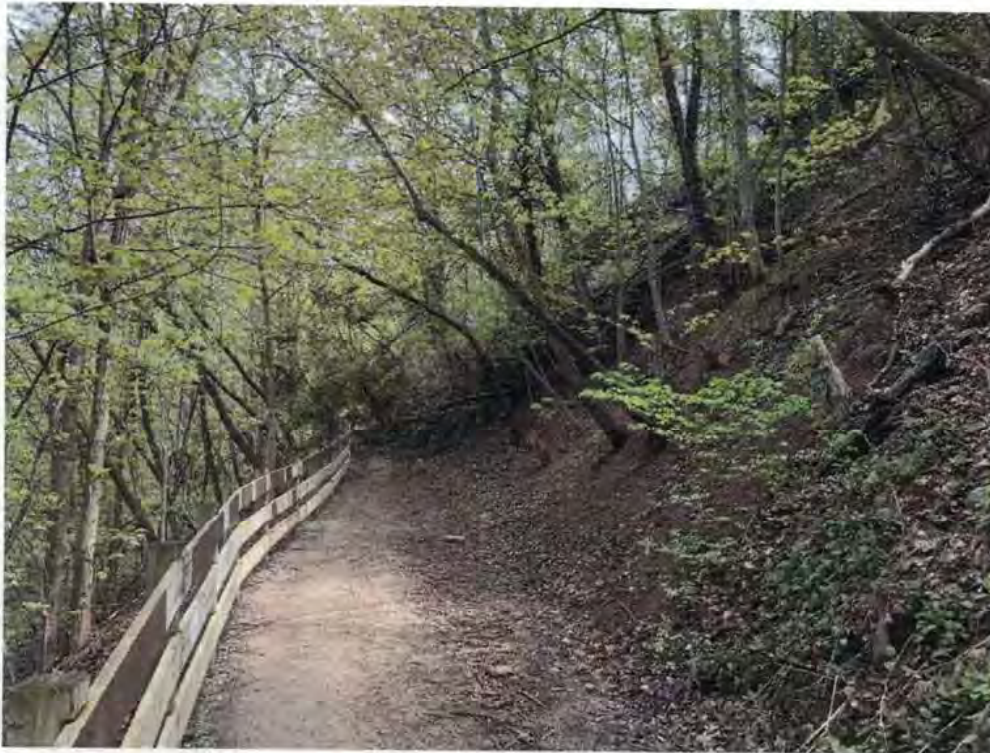
Sixteen Mile Creek Slope – Trail dividing the slope impeded by upper slope overburden erosion, looking South, Cross Section B
