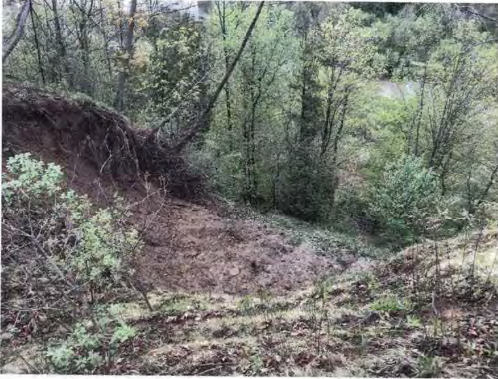
Sixteen Mile Creek Slope – Slope overburden erosion, looking East
