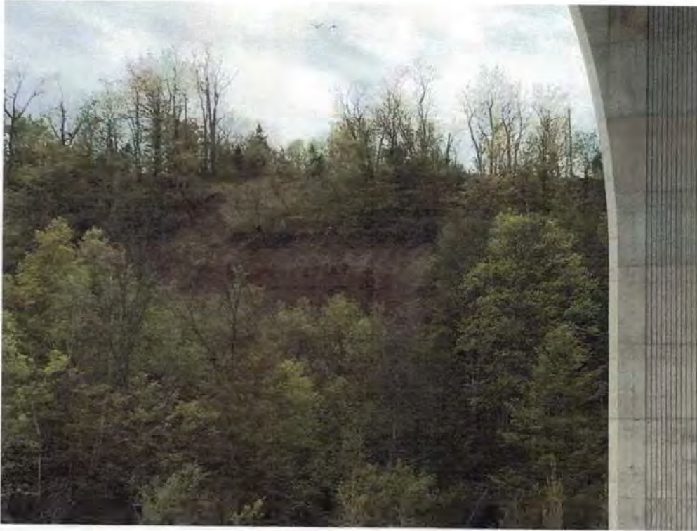
Sixteen Mile Creek Slope – Erosion of overburden on top of Queenston Shale, looking southwest, Cross Section A
