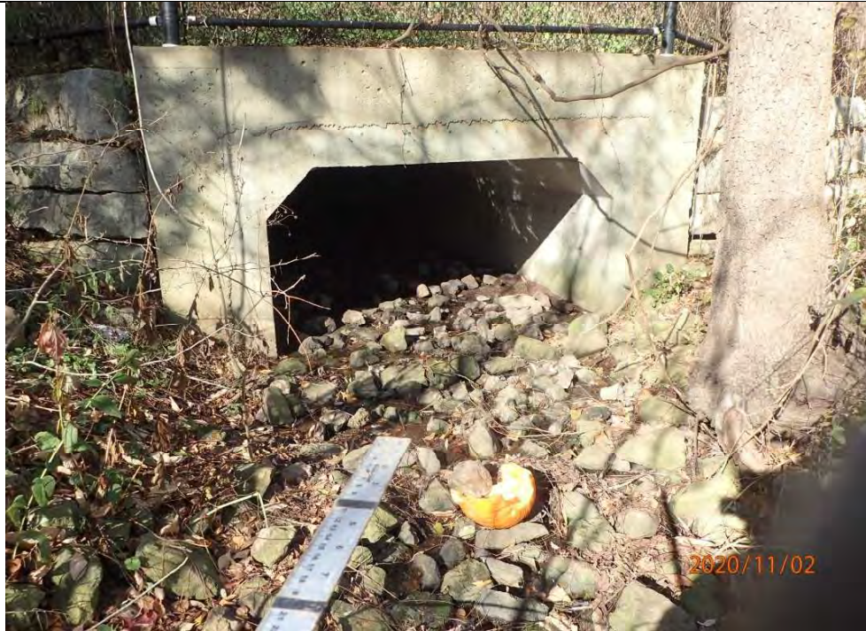
Flows exited the culvert south of Glenayr Gate into a stone treatment. No scour was noted downstream of the outlet.
