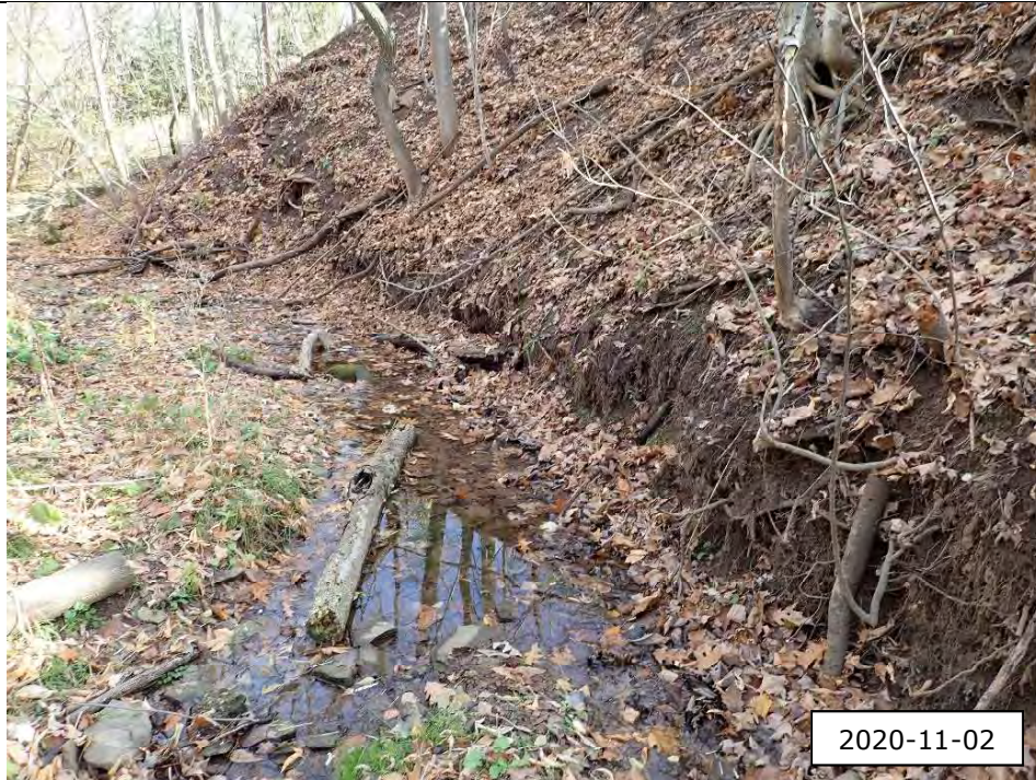
Several instances of valley wall contact and erosion were noted in Reach GC-3 .
