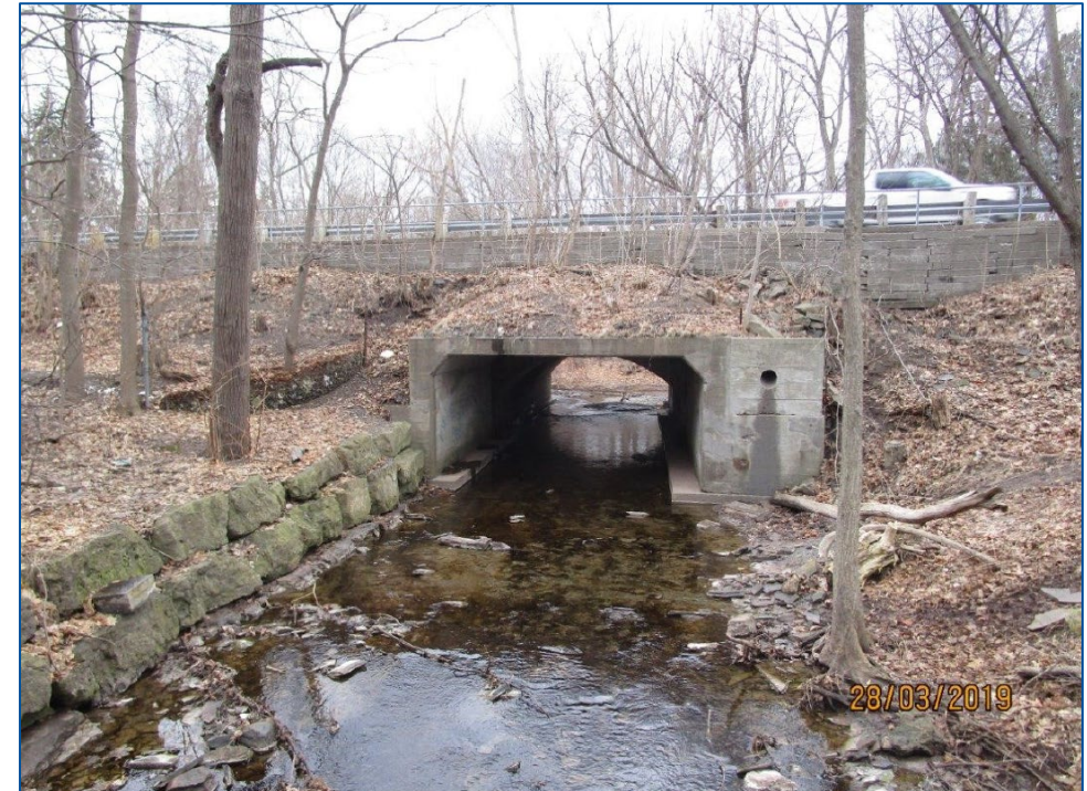
Box culvert extension of McCraney Creek Bridge along the downstream side (i.e., east side of Lakeshore Road West)
