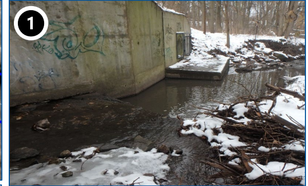
1 Vertical drop – barrier to fish passage
