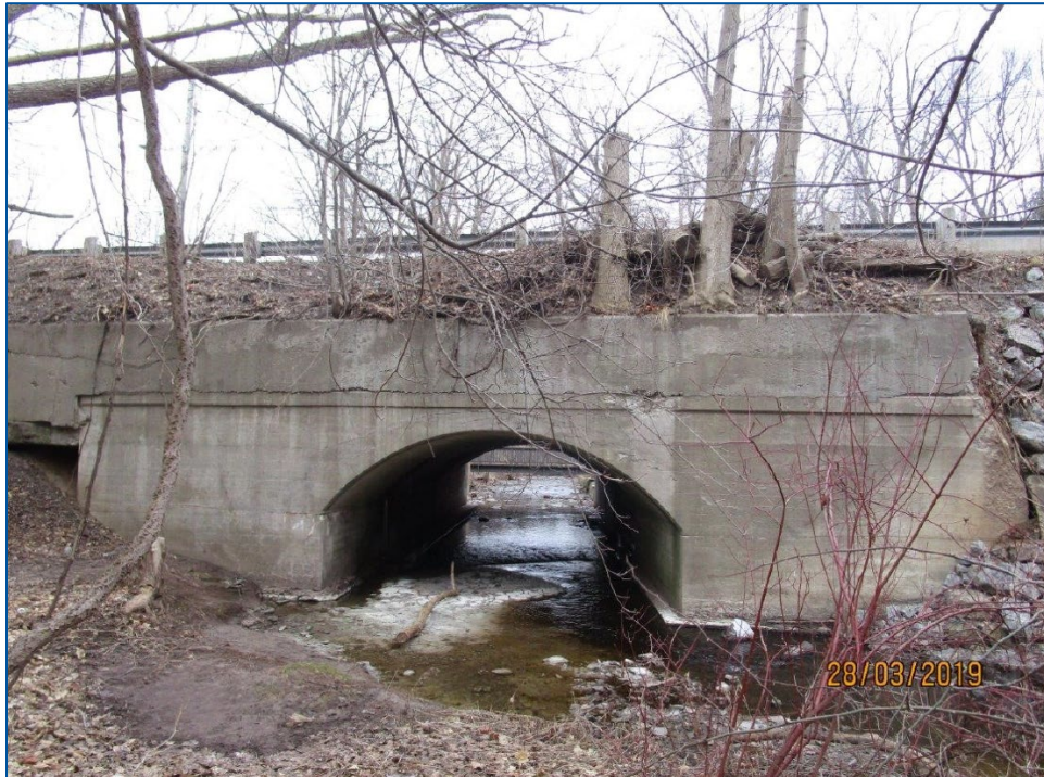
Arch structure of McCraney Creek Bridge along the upstream side (i.e., west side of Lakeshore Road West)
