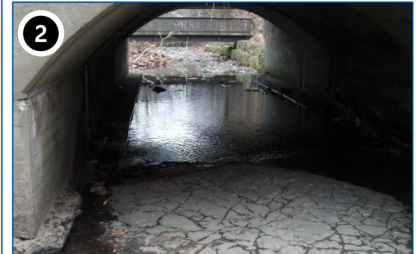
2 Exposed limestone – barrier to fish passage
