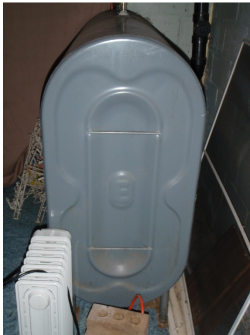
Photo 4: View of the heating oil fuel tank located in the basement of 87 Brookfield Road.
