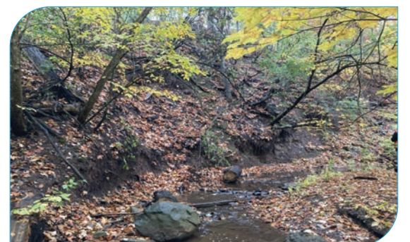
Site: E18 Score: 39 Issue: Valley wall contact; toe erosion along valley slope Risk: Pedestrian trail system; park Length: 20 – 50 m
