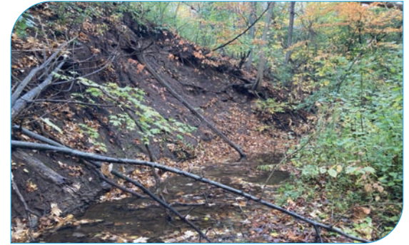
Site: E22 Score: 44 Issue: Valley wall contact; eroding valley slope Risk: Potential risk to pedestrian trail system and private property Length: 10 – 20 m
