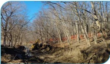
Channel to be isolated with temporary check dams and pumps to bypass creek flows
