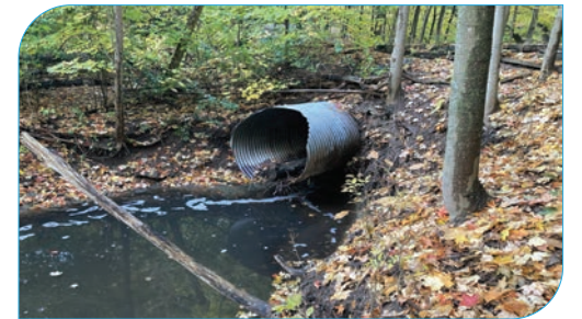
Site: E11 Score: 79 Issue: CSP culvert below trail, bottom corroded. Scour pool downstream. Buried sanitary sewer. Risk: Critical infrastructure (sanitary sewer), pedestrian path/crossing Length: 20 – 50 m
