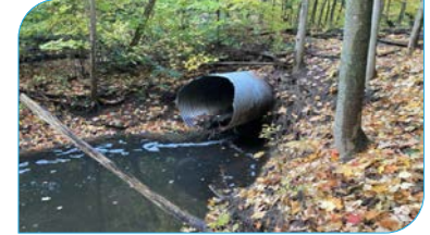
Site: E11 Score: 79 Issue: CSP culvert below trail, bottom corroded. Scour pool downstream. Buried sanitary sewer. Risk: Critical infrastructure (sanitary sewer), pedestrian path/crossing Length: 20 – 50 m
