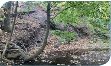
Site: E7, E9 Score: 56, 53 Issue: Toe erosion of valley slope (unprotected) Risk: Private property (parking lot) Length: 10 – 20 m
