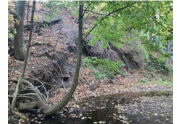
E7: Toe erosion of valley slope. Risk to private properties (parking lot) at top of slope.
