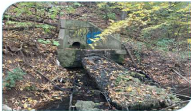
Site: E6 Score: 64 Issue: Perched outfall on valley slope, outfall drop structure suspended, scour pool below Risk: Private property; secondary infrastructure (outfall) Length: 50 – 100 m
