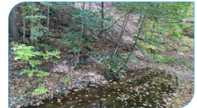
Site: E24 (new site) Score: 59 Issue: Valley contact/slope erosion. Gabion toe protection - fair condition (functioning, some wire failure at toe) Risk: Private property Length: 20 – 50 m
