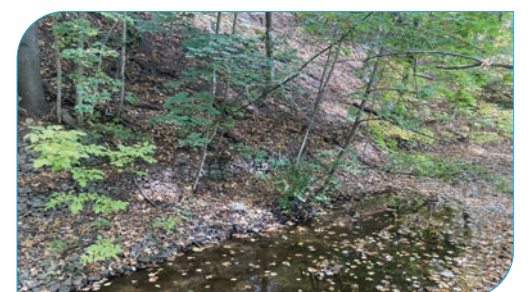
Site: E24 (new site) Score: 59 Issue: Valley contact/slope erosion. Gabion toe protection - fair condition (functioning, some wire failure at toe) Risk: Private property Length: 20 – 50 m
