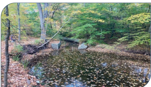
Site: E5 Score: 51 Issue: Gabion baskets lining both banks. Failing at downstream end and large scour pool. Risk: Secondary infrastructure (gabion baskets), pedestrian trail Length: 20 – 50 m
