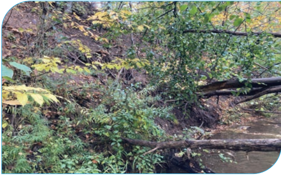
Site: E23 Score: 37 Issue: Valley wall contact; eroding valley slope Risk: Potential risk to pedestrian trail system and private property Length: 10 – 20 m
