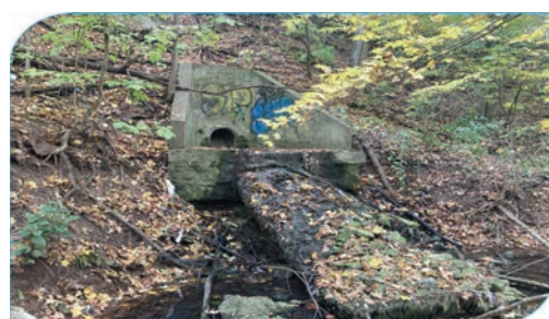
Site: E6 Score: 64 Issue: Perched outfall on valley slope, outfall drop structure suspended, scour pool below Risk: Private property; secondary infrastructure (outfall) Length: 50 – 100 m
