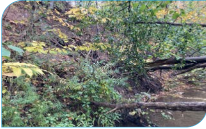
Site: E23 Score: 37 Issue: Valley wall contact; eroding valley slope Risk: Potential risk to pedestrian trail system and private property Length: 10 – 20 m
