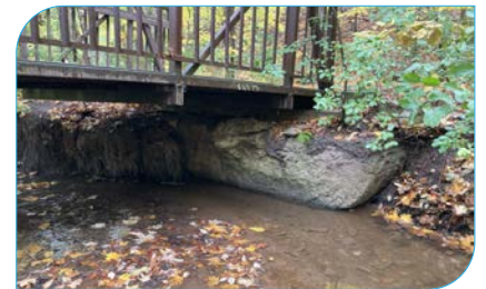
Site: E20 Score: 43 Issue: Erosion around pedestrian bridge crossing; footing exposed on the outer meander bend. Risk: Trail infrastructure including pedestrian trail and pedestrian bridge crossing Length: < 10 m
