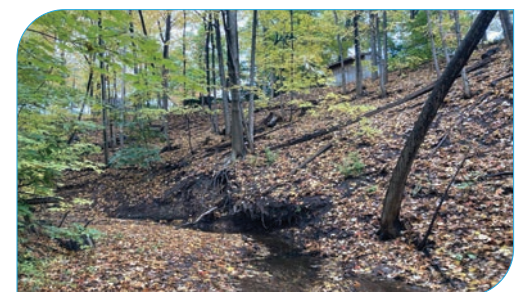
Site: E10 Score: 60 Issue: Erosion at toe of valley slope in tributary (unprotected); private property at top of slope. Risk: Private property Length: 10 – 20 m
