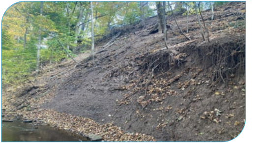
Site: E4 Score: 65 Issue: Valley wall contact and slope erosion. Gabion protection near upstream end of erosion is in poor condition (bottom tier corroded/emptied) Risk: Private property Length: > 100 m
