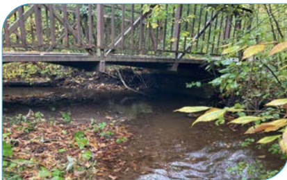
Site: E21 Score: 43 Issue: Erosion around pedestrian bridge; footing exposed within the channel. No damage to the concrete footing currently. Risk: Trail infrastructure including pedestrian trail and pedestrian bridge crossing Length: < 10 m
