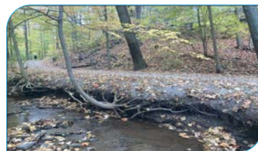
Site: E1, E2, E3, E8, E12, E13 (not included in EA) Score: 35, 26, 34, 38, 42, 43 Issue: Bank erosion in proximity to pedestrian trail system; not valley contacts. Risk: Mainly pedestrian trail system, pedestrian bridge (E13), secondary infrastructure (stormwater outfall - E12) Length: varies
