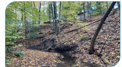
Site: E10 Score: 60 Issue: Erosion at toe of valley slope in tributary (unprotected); private property at top of slope. Risk: Private property Length: 10 – 20 m
