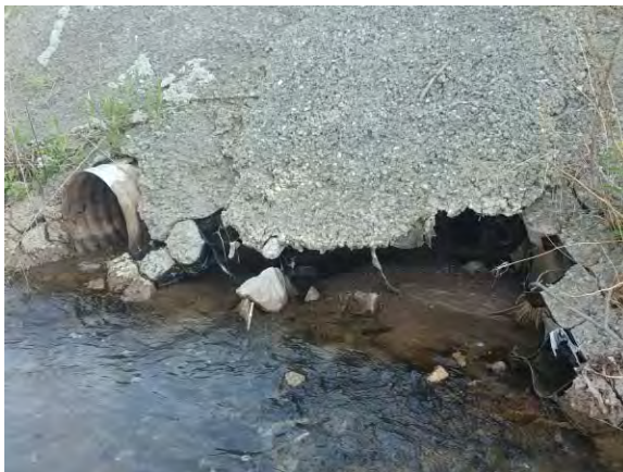
Photo 15: Eroding channel banks (up to 90 cm undercut), located within 6m downstream of the Wyecroft Rd. culvert.
