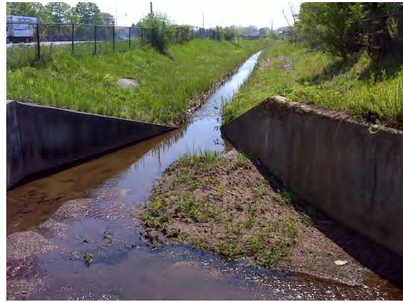
Photo 27: Downstream view of channel showing widened outlet area and depositional area.
