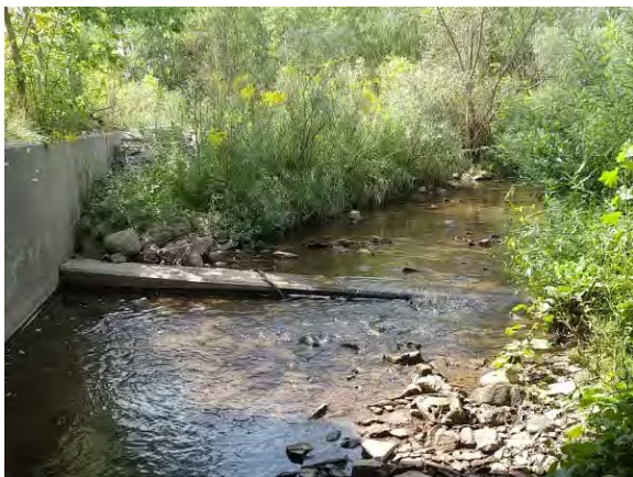
Photo 11: Upstream view of concrete lip at the inlet of the culvert (September 7, 2018).
