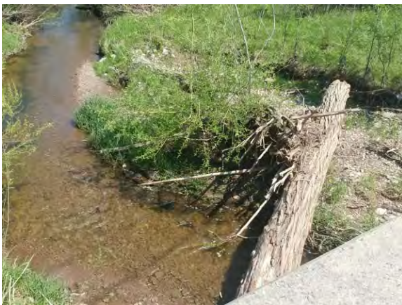
Photo 5: View from on top of the structure outlet, showing large log across channel.
