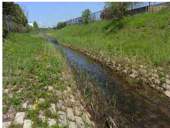
Photo 29: Upstream view of downstream channel reach (concrete blocks on bank and in channel visible); some instream vegetation present.
