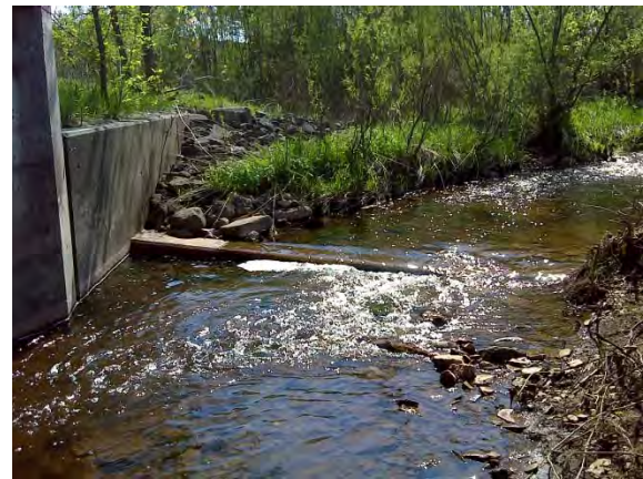
Photo 4: Concrete lip located at structure inlet; partially exposed above the water at the time of survey (May 17, 2018).
