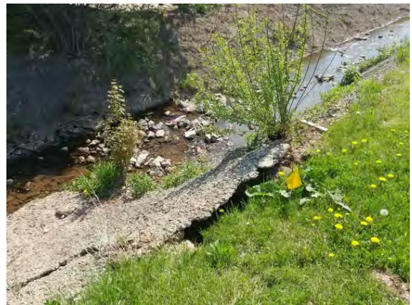
Photo 14: Eroding concrete channel banks near the culvert outlet.
