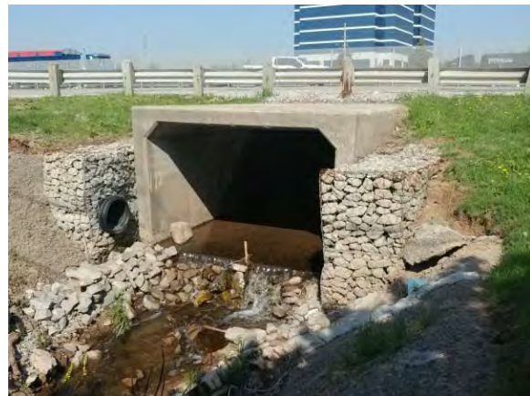
Photo 16: Upstream view of the culvert outlet, highlighting perch (May 17, 2018).
