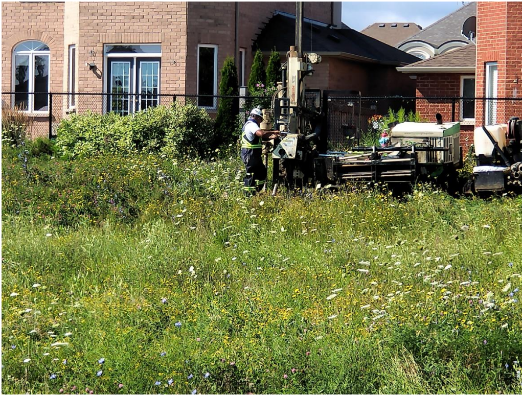
Photograph No. 3 – View of the advancement of borehole BH102-21 within the western soil berm.
