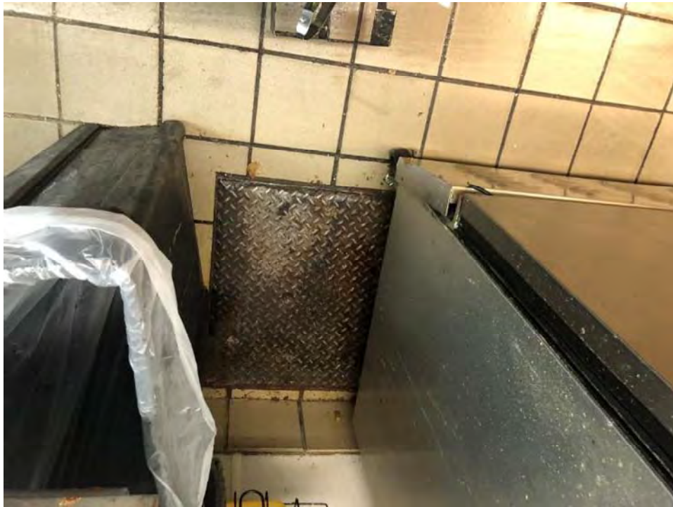
Photo 7: Grease trap located at the north portion of the Site building.
