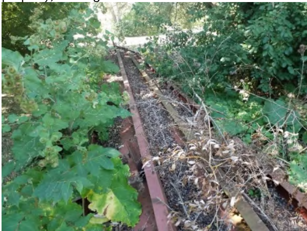
Plate 11: Metal beams and debris on ground surface in the northwestern area of the property, looking south.
