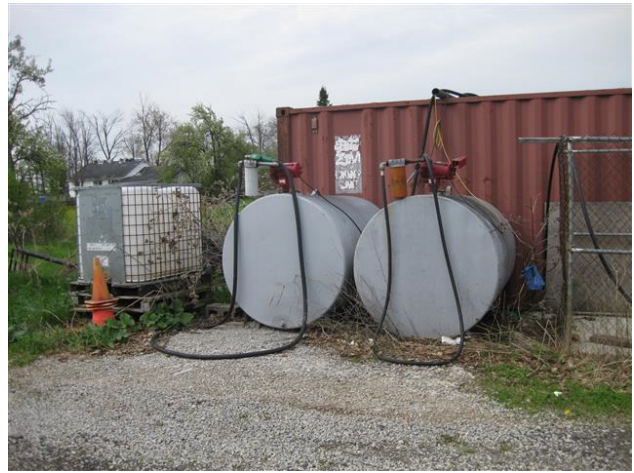
Photo 10: View of the aboveground storage tanks (ASTs) on the west adjacent property.
