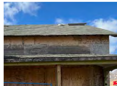
View of asphalt shingles in poor condition (ERA, 2023).
