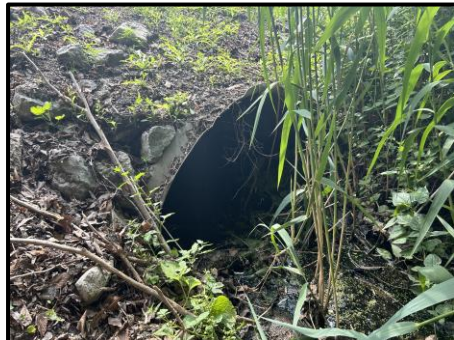
Culvert Face Showing Standing Water and Sedimentation
