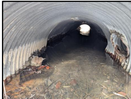
Visible Corrosion Within Culvert
